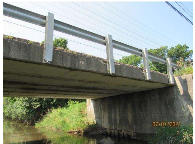
Spalling Along North Coping
