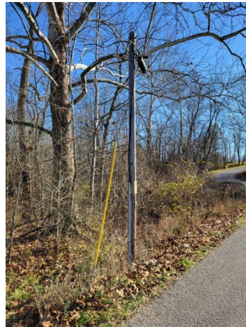
Centurylink Underground/Overhead Transition South of Bridge 56
