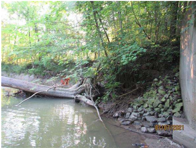
Heavy Bank Erosion (Southeast Corner)
