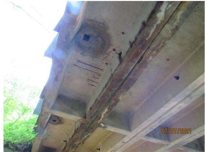
Exposed Steel in Beam 1
