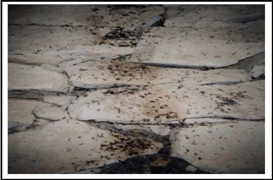
9-1.6 Bat Guano on Riprap
