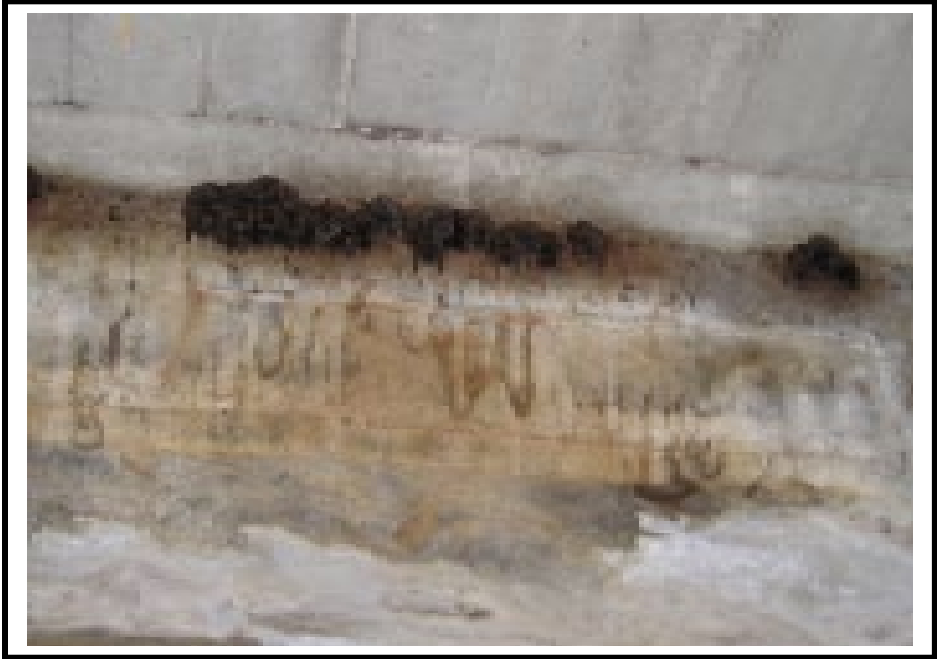
9-1.5 Bats Roosting Along Crack and Associated Staining
