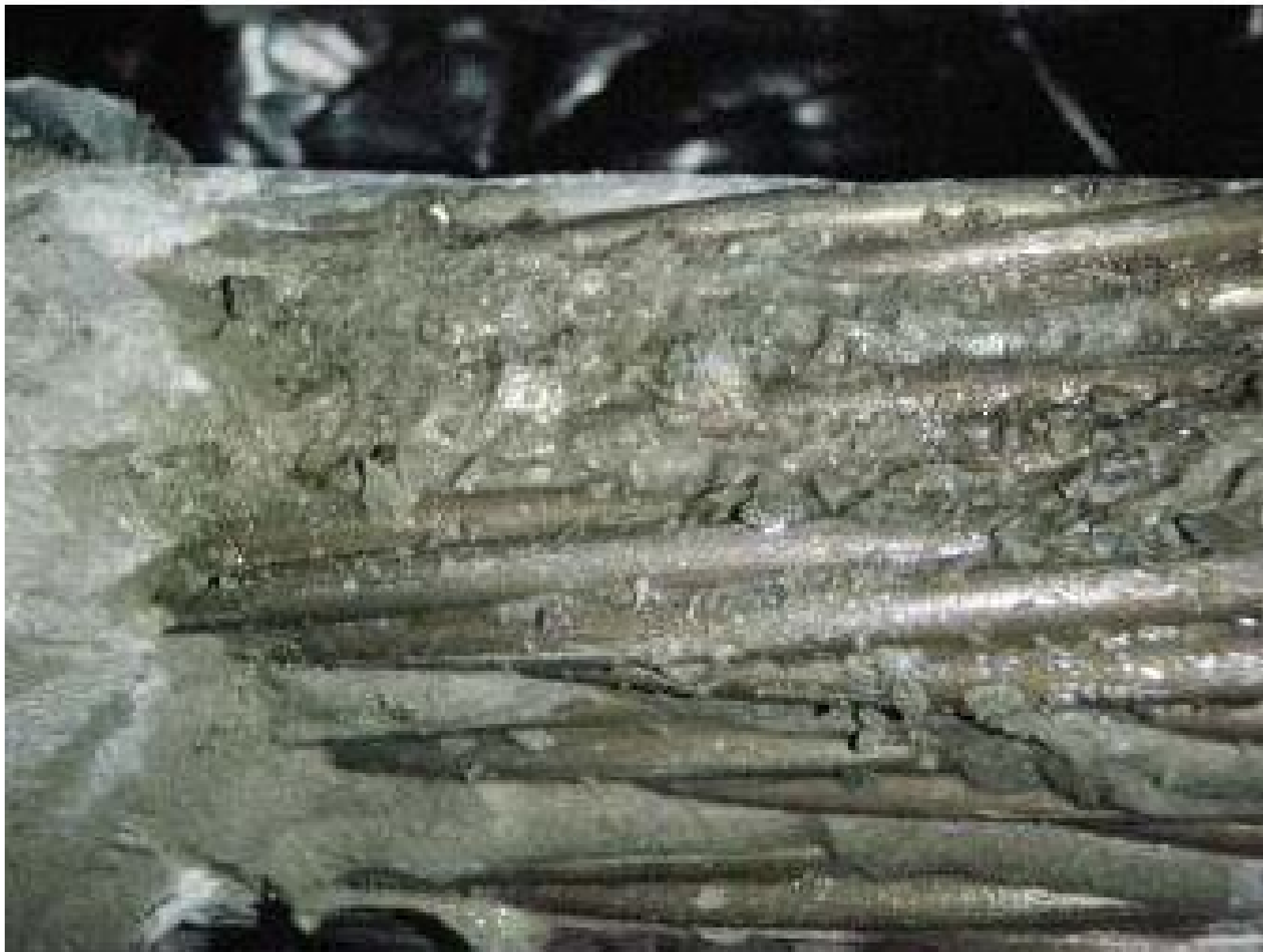
Post-Tech CI material clearly visible in the strands as well as the surrounding grout
