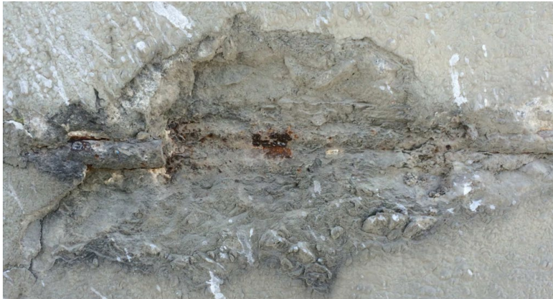
Low / no cover of Reinforcing Steel
