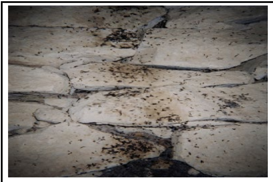
9-1.6 Bat Guano on Riprap
