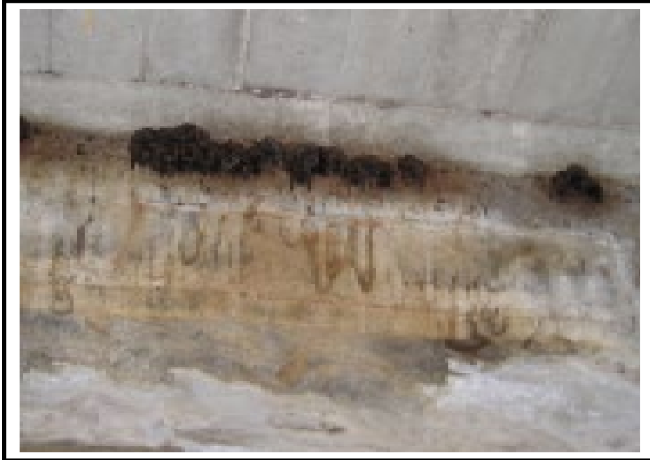
9-1.5 Bats Roosting Along Crack and Associated Staining
