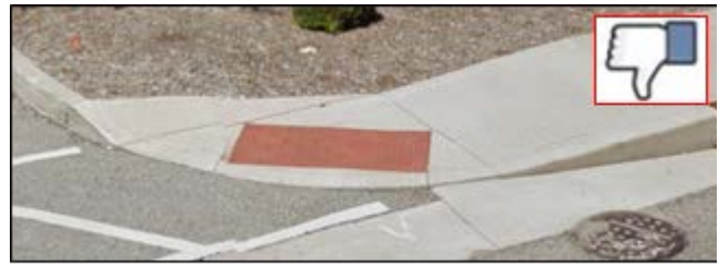
Detectable Warning Surface is not full width of the ramp. See below for possible solutions.
