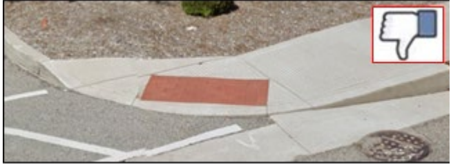
Detectable Warning Surface is not full width of the ramp. See below for possible solutions.
