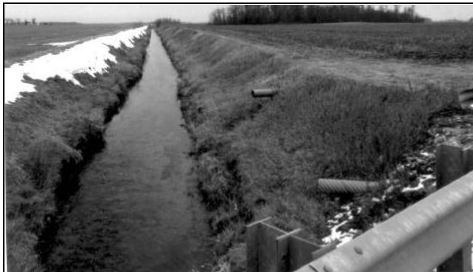
Exhibit 1001a: A Tile Drain Outlet Extension (Source: Tipton County Files)
