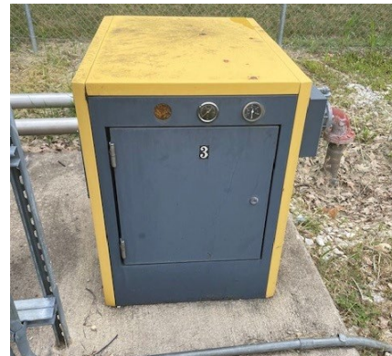
Blower #3 – Not in Service
