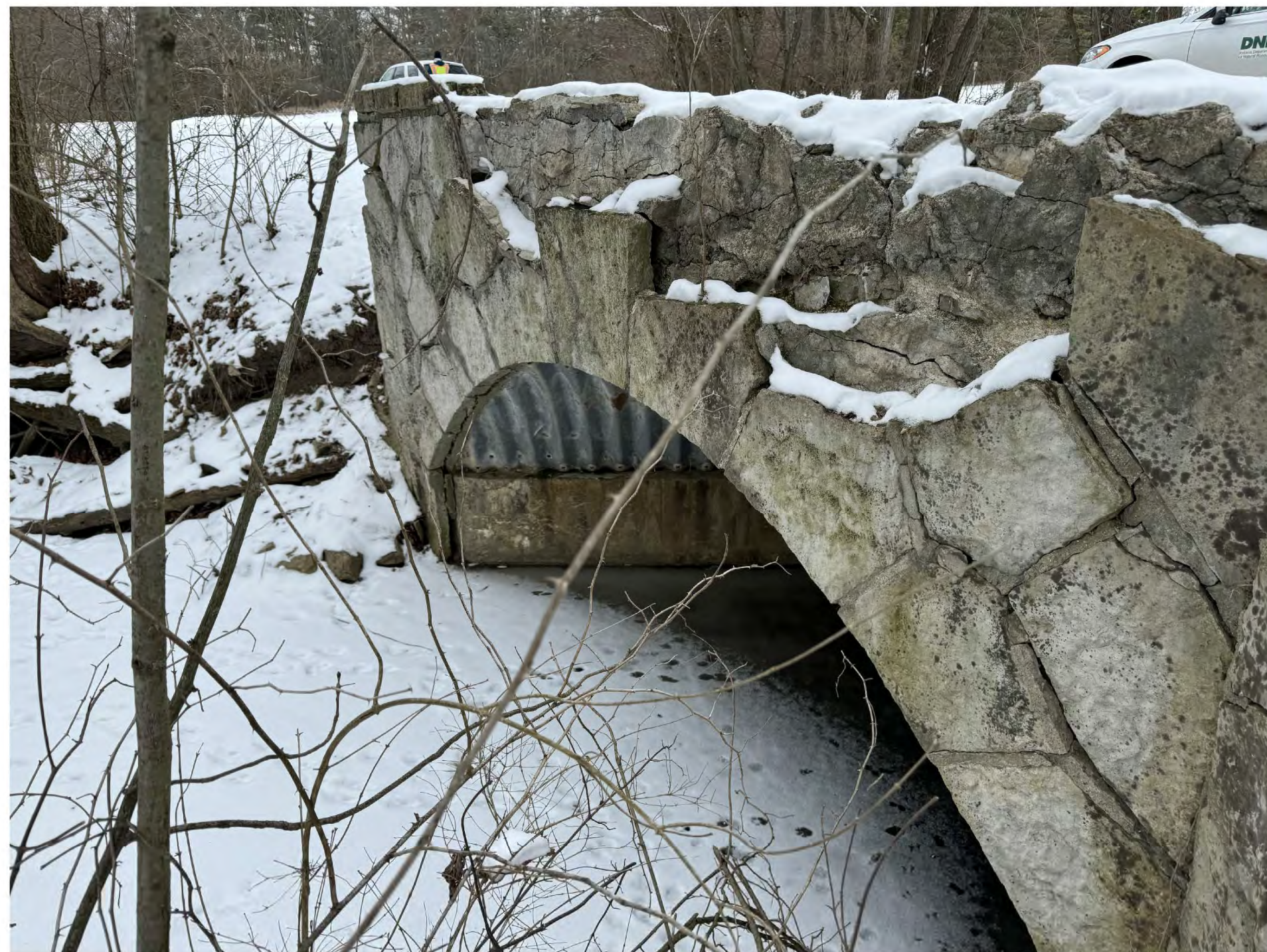
4. Side elevation at the upstream. Stone to be removed, salvaged, cleaned and reset.
