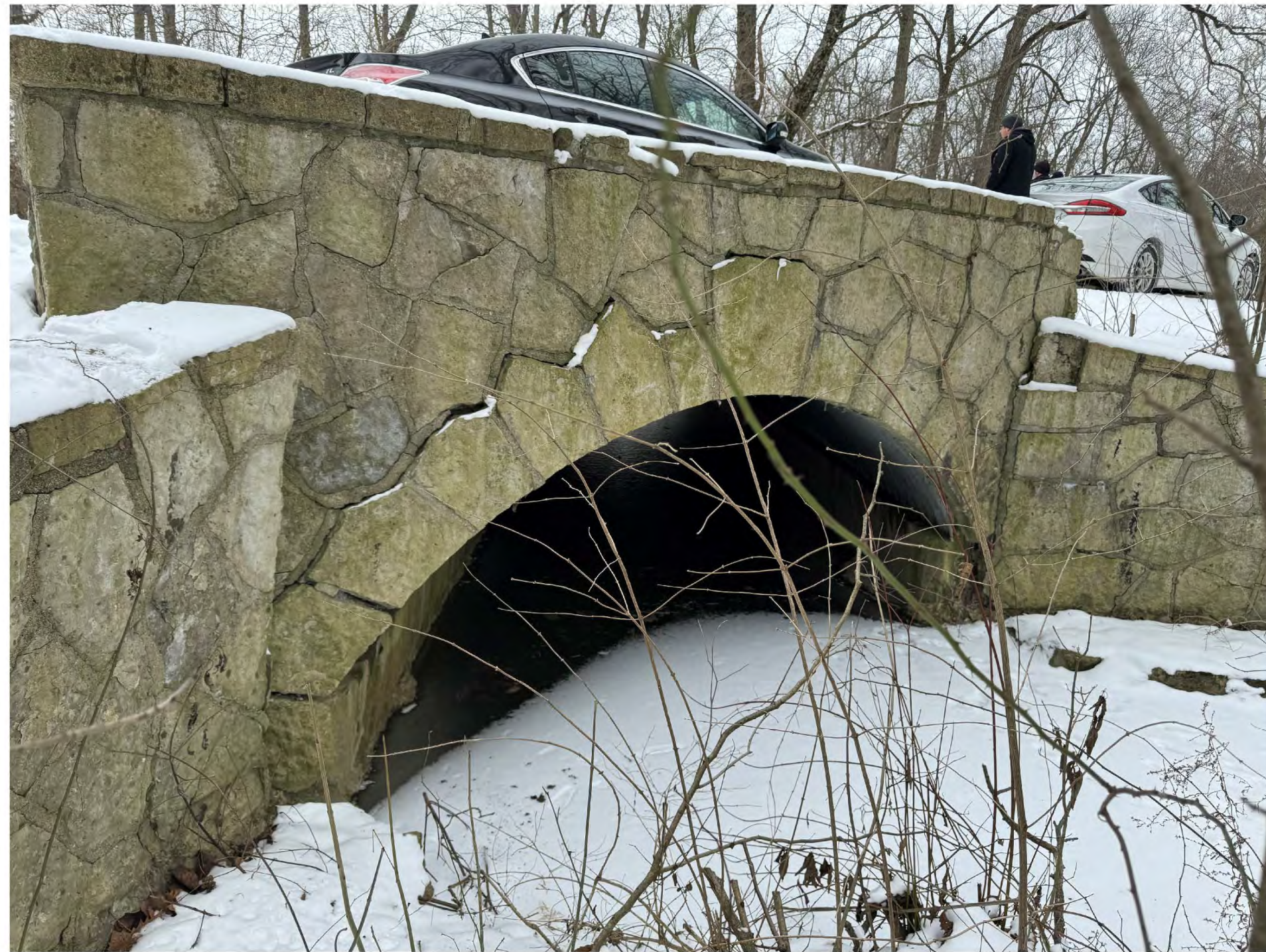
1. Side elevation at the downstream. Stone to be removed, salvaged, cleaned and reset.
