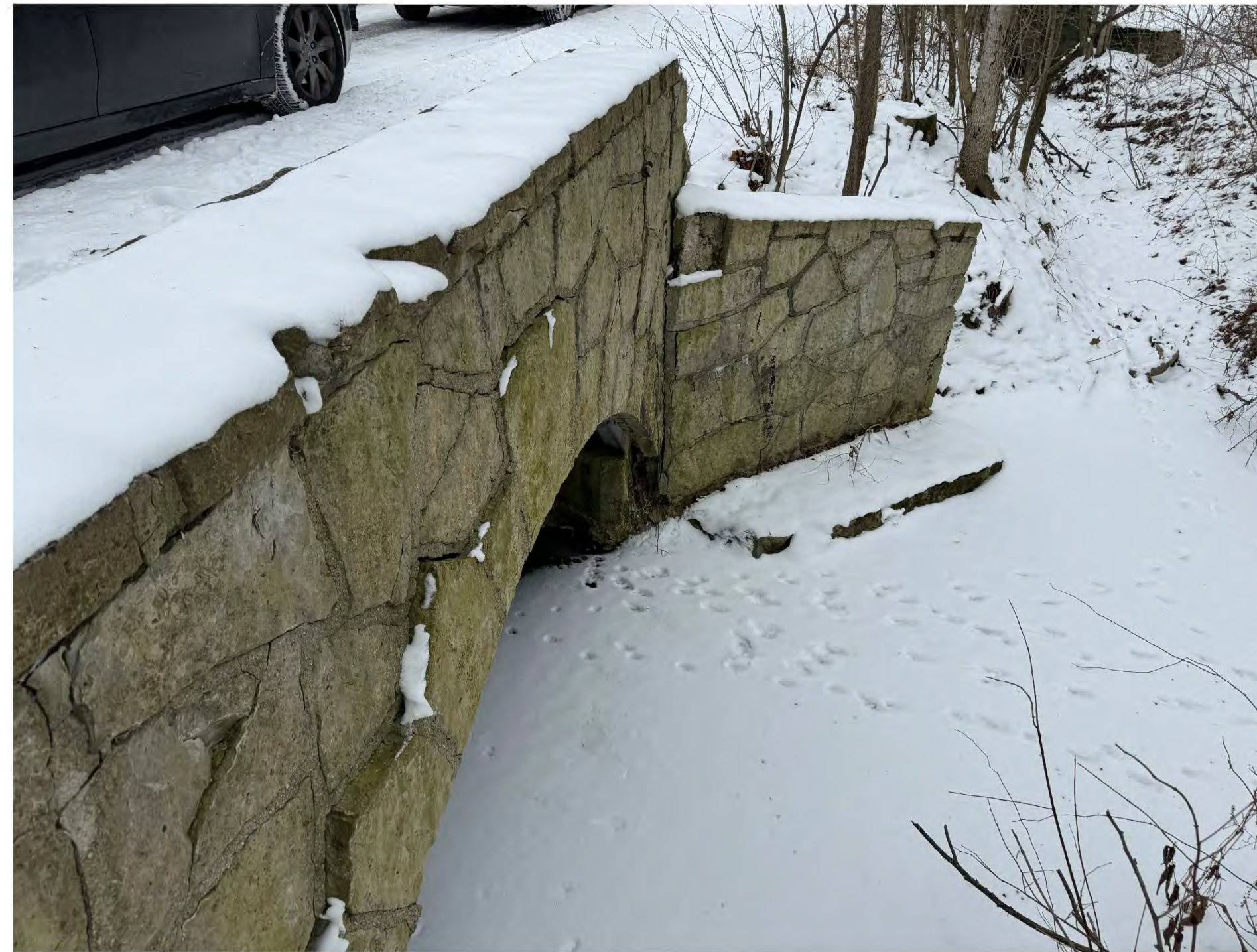
2. Side elevation at the downstream. Stone to be removed, salvaged, cleaned and reset.
