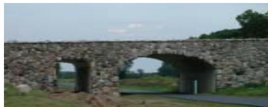
The stone bridge, built of locally gathered stone, provides a study of the local geology.
