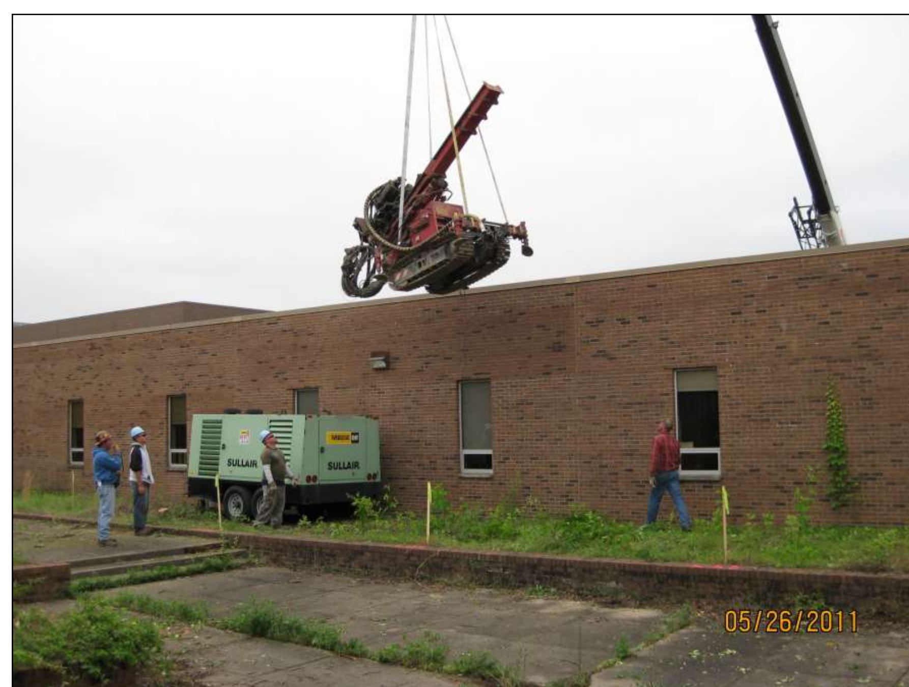
To utilize the central courtyard, the drilling equipment was lifted over the building using a large crane.
