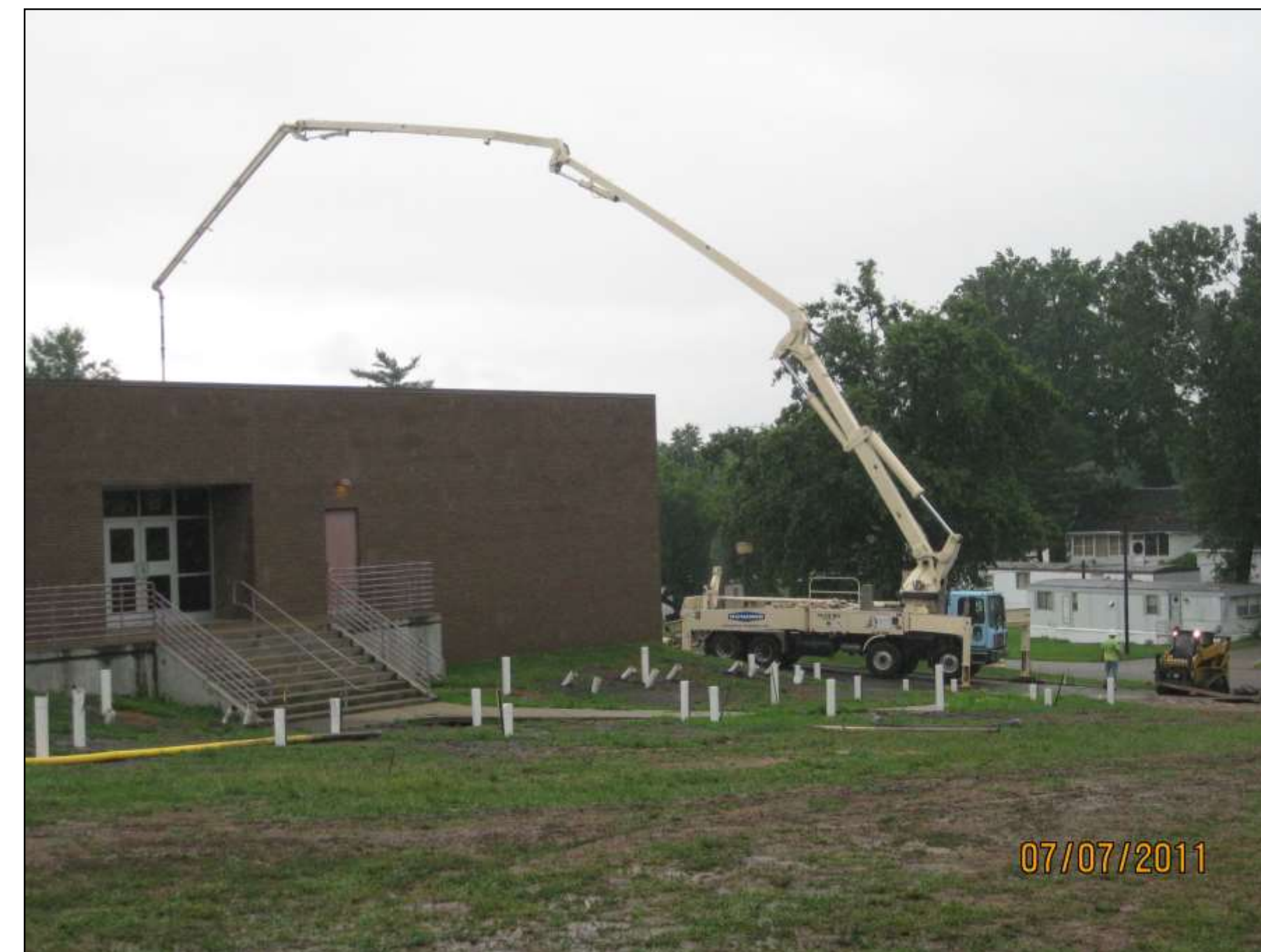
Grout was pumped from the building perimeter using a pump truck with large articulated pumping booms.
