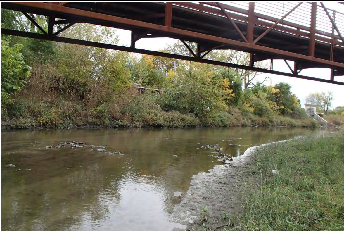
Existing Monon Trail Pedestrian Bridge over the Little Calumet River, facing northeast.
