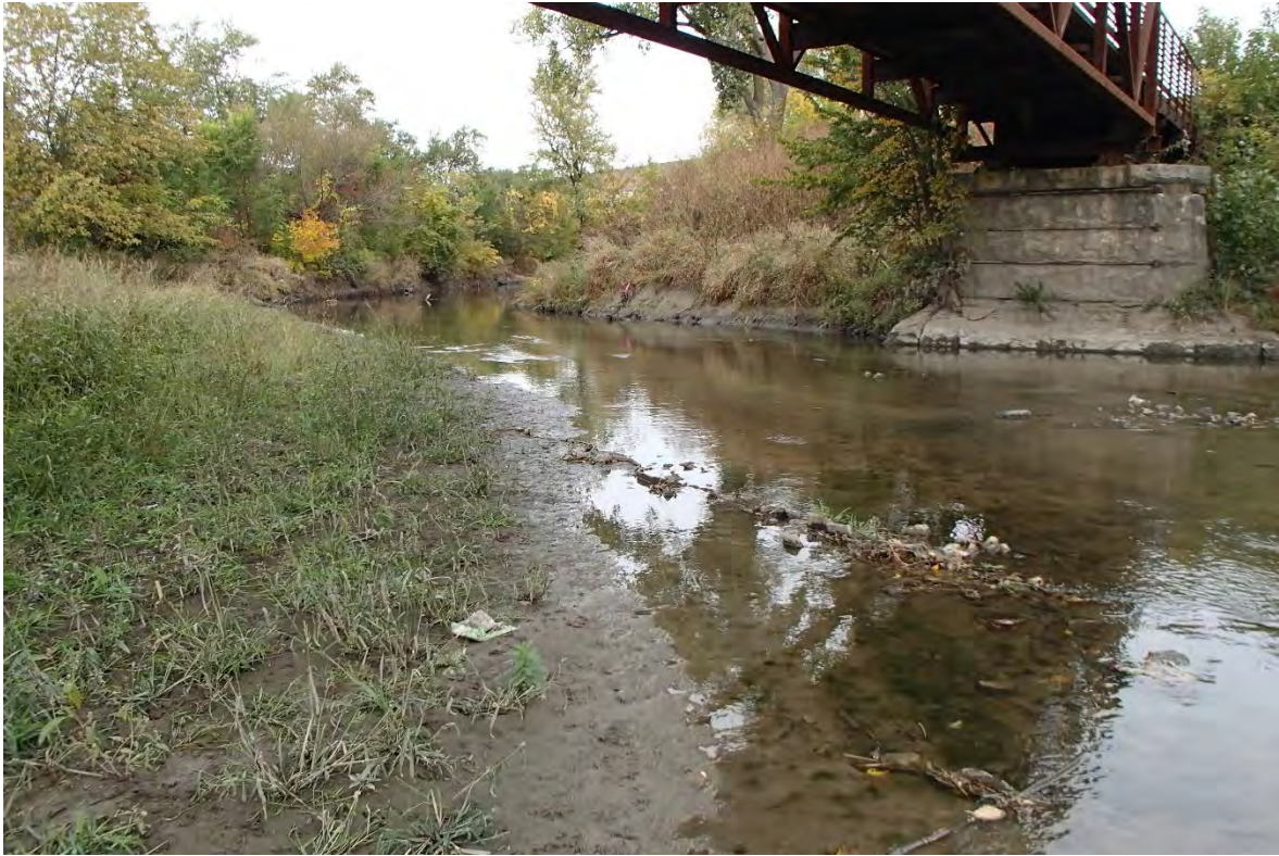
Existing Monon Trail Pedestrian Bridge over the Little Calumet River, facing northwest.
