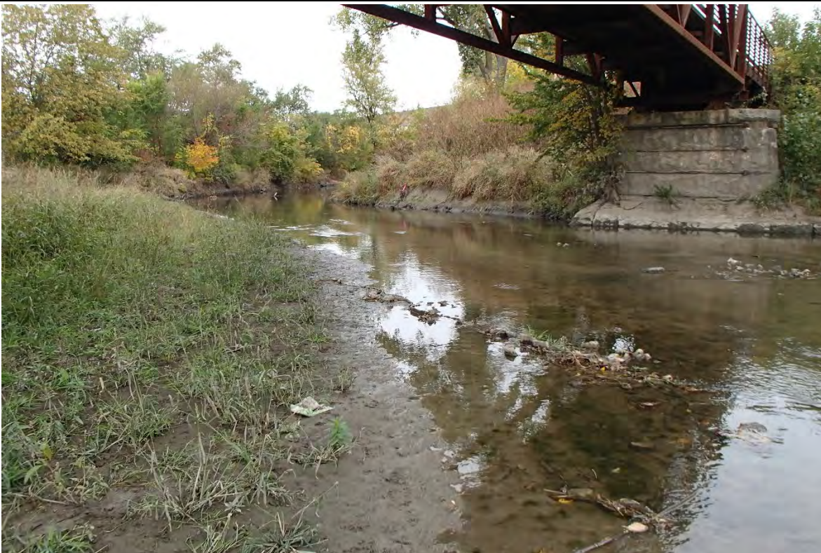
Existing Monon Trail Pedestrian Bridge over the Little Calumet River, facing northwest.
