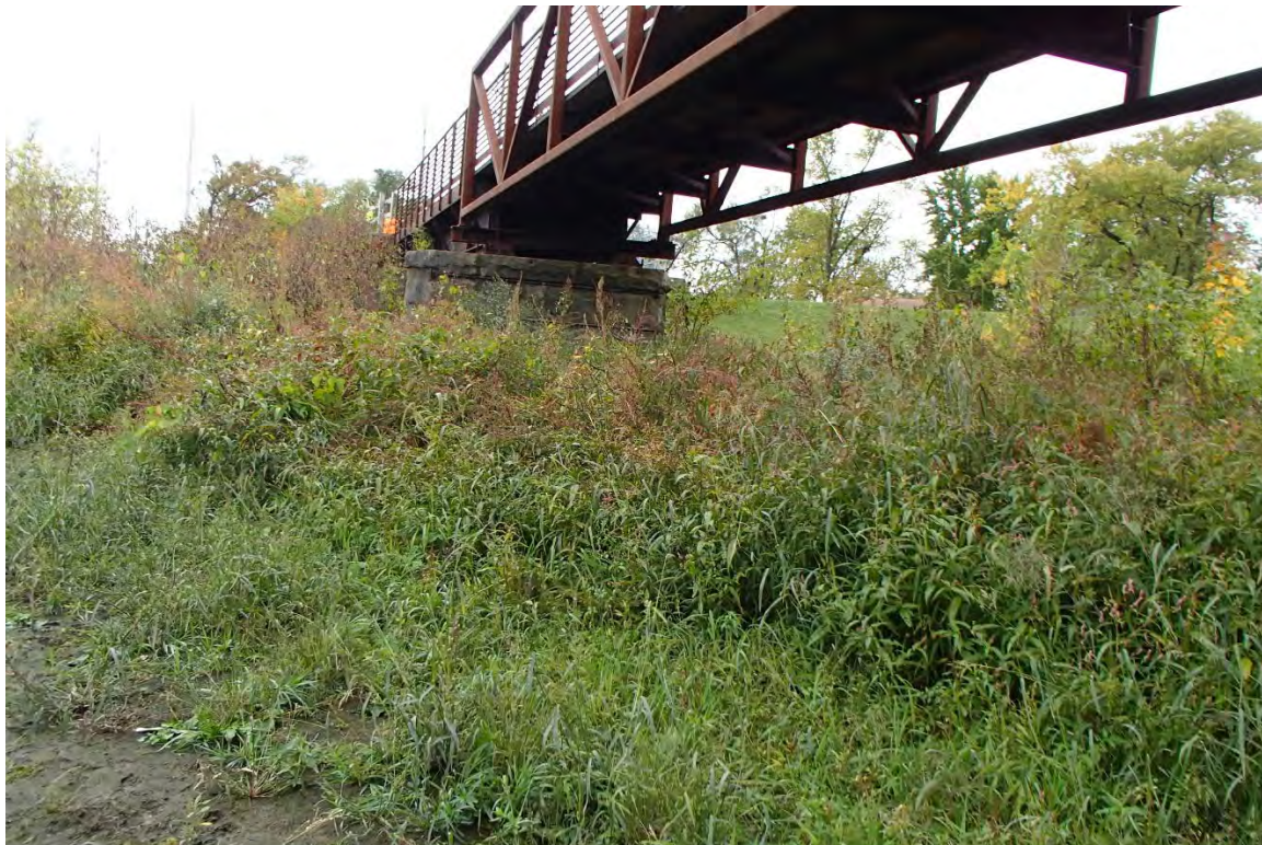
Existing Monon Trail Pedestrian Bridge over the Little Calumet River, facing south.
