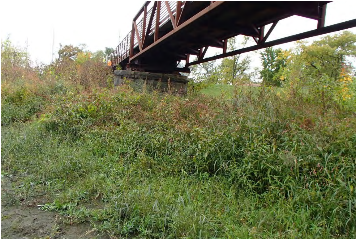
Existing Monon Trail Pedestrian Bridge over the Little Calumet River, facing south.
