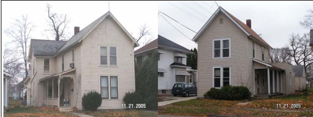
Look at your surroundings, often a neighboring building reveals clues to your building's character. These two houses in the Drover Town Historic District, Huntington, Indiana, were likely very similar at one point. The house at left would assess at a higher value due to the wing. Photos by John Warner.
