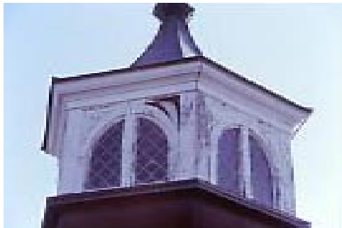
The deteriorated cupola of the Christamore House. (Photo DHPA).
