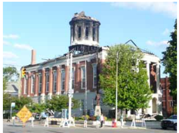
A street view of the Jefferson County Courthouse after the fire. (Photo DHPA).
