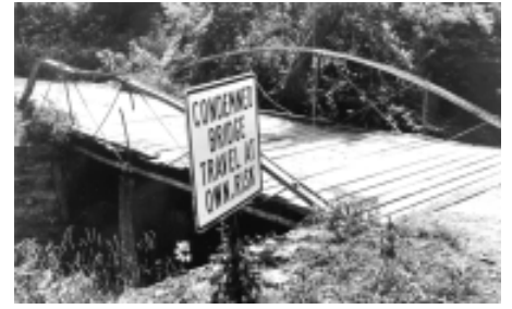
This small county bridge's trusses have suffered serious damage.
