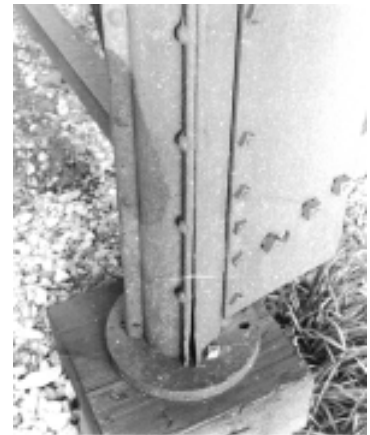
The Phoenix Column is an example of a patented element found on some metal truss bridges.
