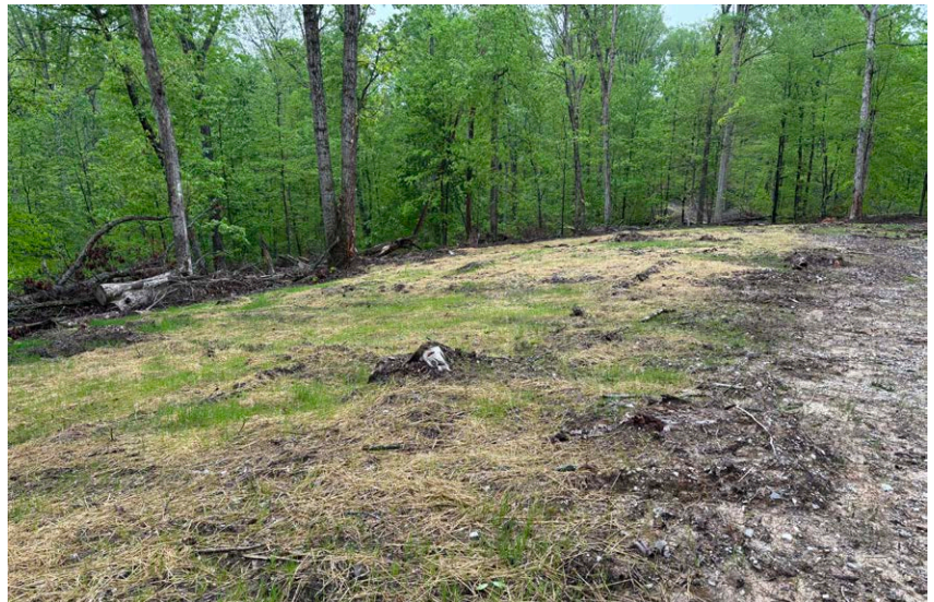
While this landing is on a fairly steep slope, it has been smoothed, mulched, and seeded, with debris placed on the downslope side to slow and filter runoff. Photo taken on state property by Jennifer Sobecki, DNR.
