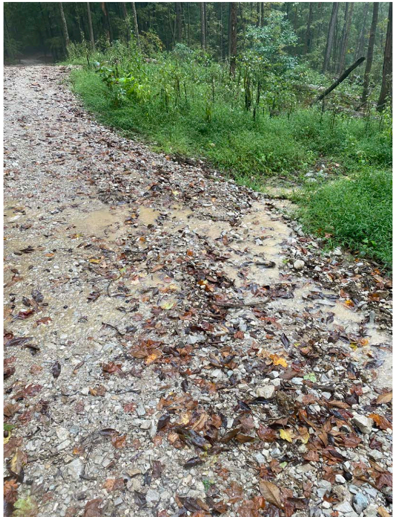
An outslope & cut out work to move runoff of an access road onto forest floor where it can be absorbed. Photo taken on state forest property by Duane McCoy, DNR.
