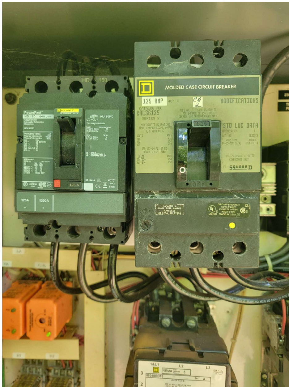
Photograph No. 3 – Sunset Point Lift Station – Base Bid
