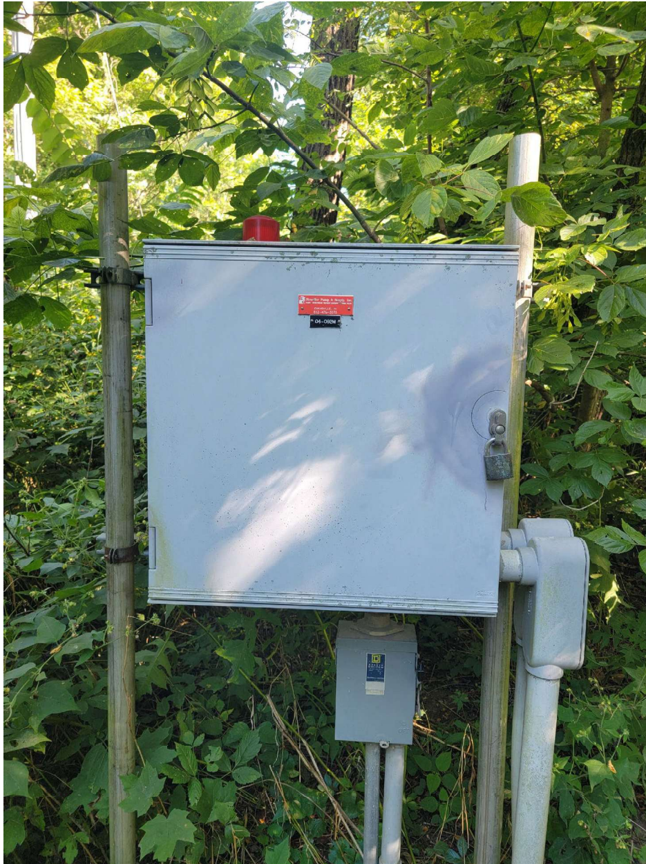
Photograph No. 5 – West Campground Lift Station – Alternate #1
