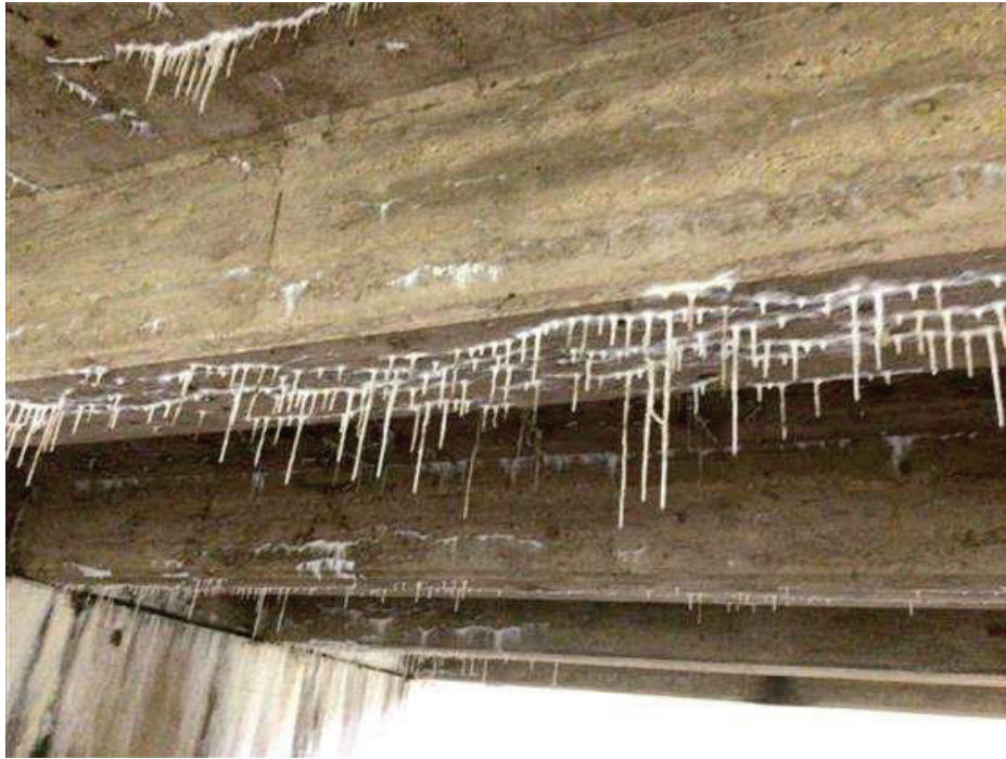
PHOTO 17 Condition Description Span f
