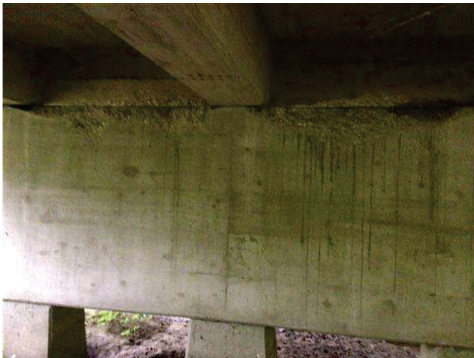
PHOTO 14 Condition Description Spalling on pier 4
