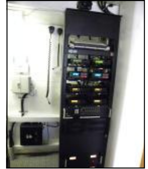
Operations inside of a Mobile Command Center
