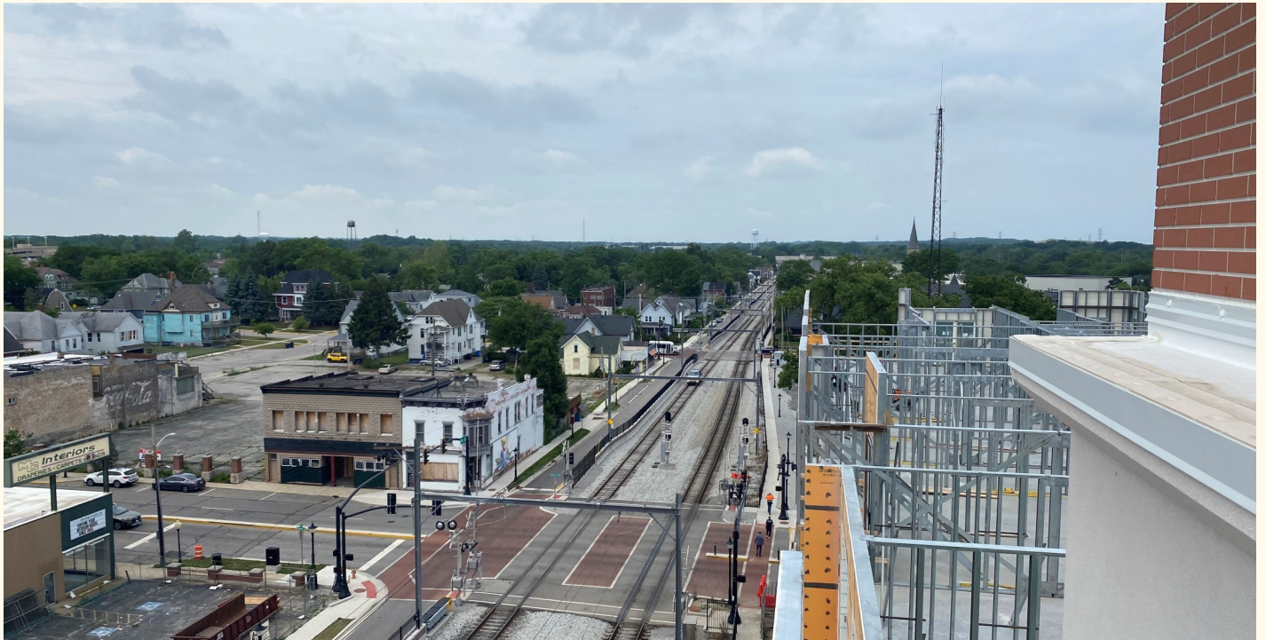
The now double-tracked main South Shore line headed west toward Chicago, as seen from the roof of the 11th Street Station parking garage in Michigan City. The metal framing on the lower right of the photo is the ongoing construction of the $101 million Franklin Tower apartments, part of the more than half a billion dollars in Transit-Oriented Development already underway as a result of the Double Track and West Lake projects.
