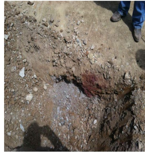
(b) Poorly mixed lime-soil modified soil
