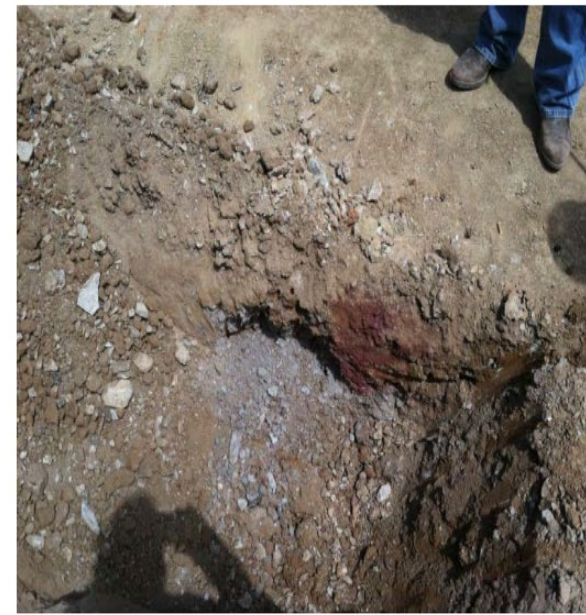
(b) Poorly mixed lime-soil modified soil
