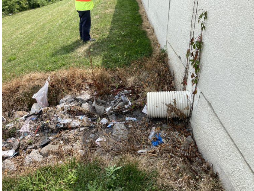
Figure 11: Blocked MSE wall drain
