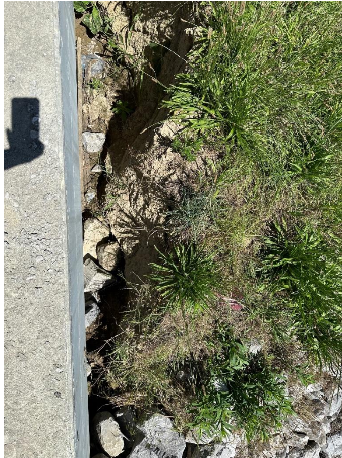
Figure 2: Erosion at the back face of the wall
