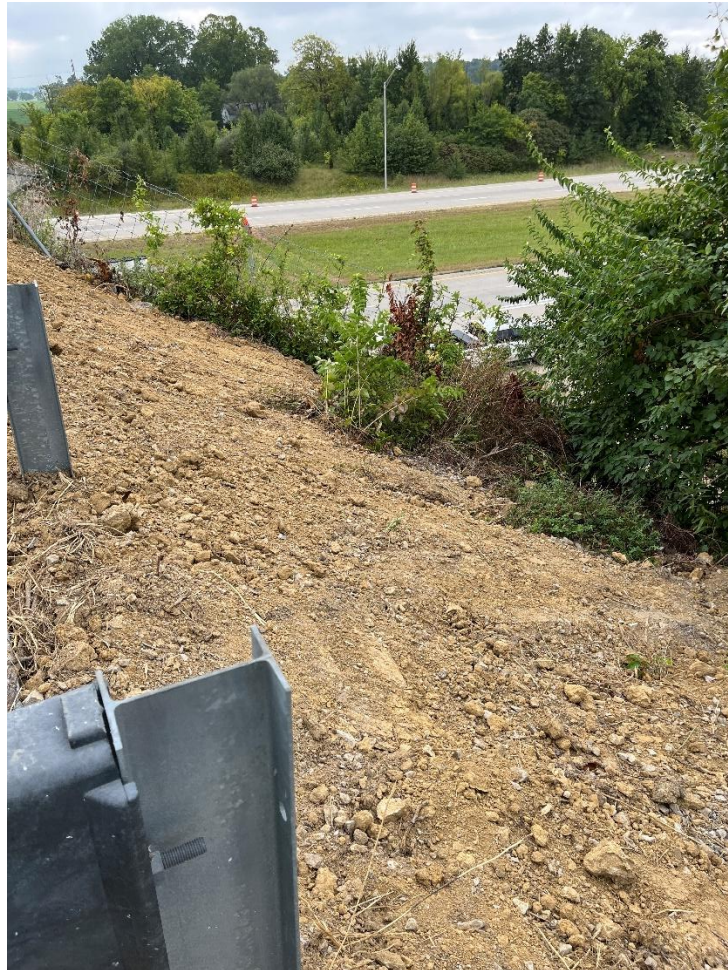
Figure 3: Recompacted eroded backfill of MSE wall
