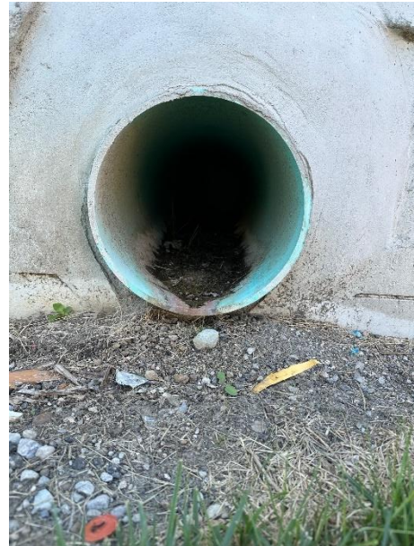
b) Clogged pipe
