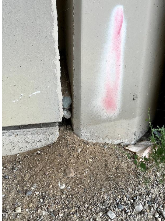
Figure 6: Soil leaking through wide panel joints
