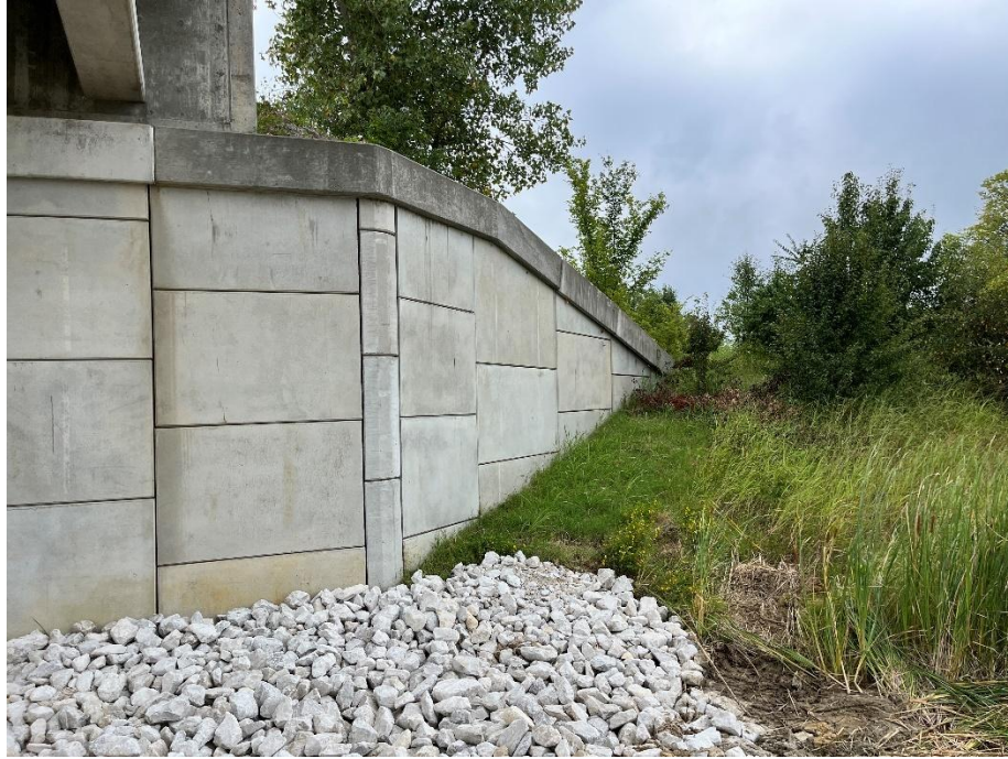
Figure 5: Grown tree on top of the MSE wall
