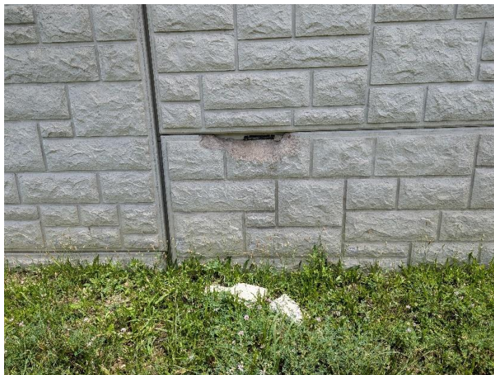
Figure 7: Spalling in the concrete panel
