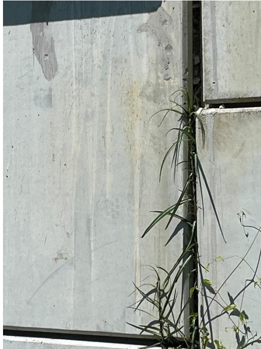
Figure 4: Vegetation growing through panel joints
