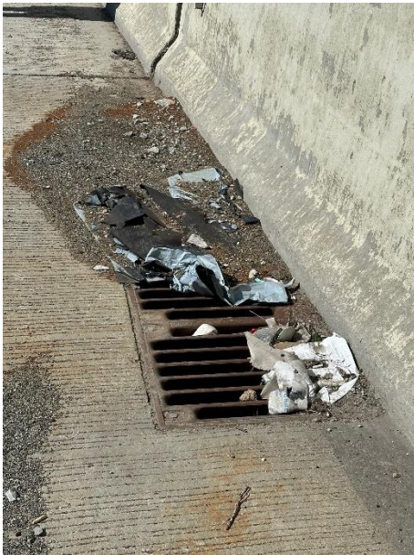
a) Clogged manhole
