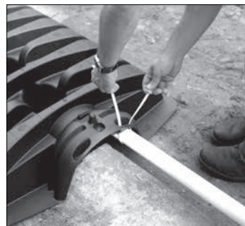
5. Secure pressure pipe.
