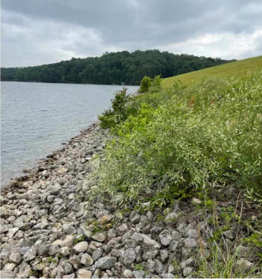
Brush to be removed along embankment.
