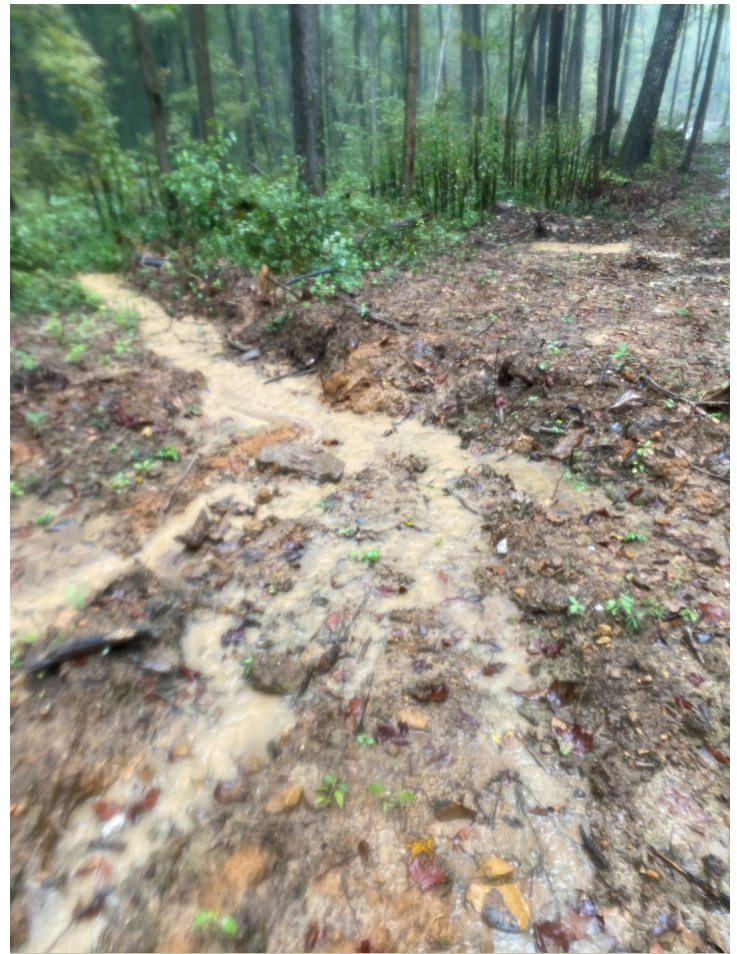
Waterbars doing their job during a rainstorm. Photo by Duane McCoy, DNR
