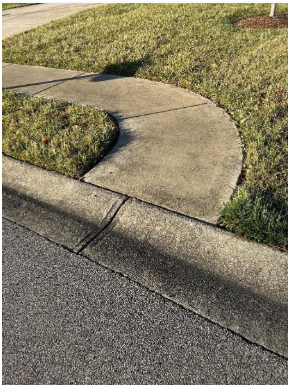
Missing curb ramp at the northwest end
