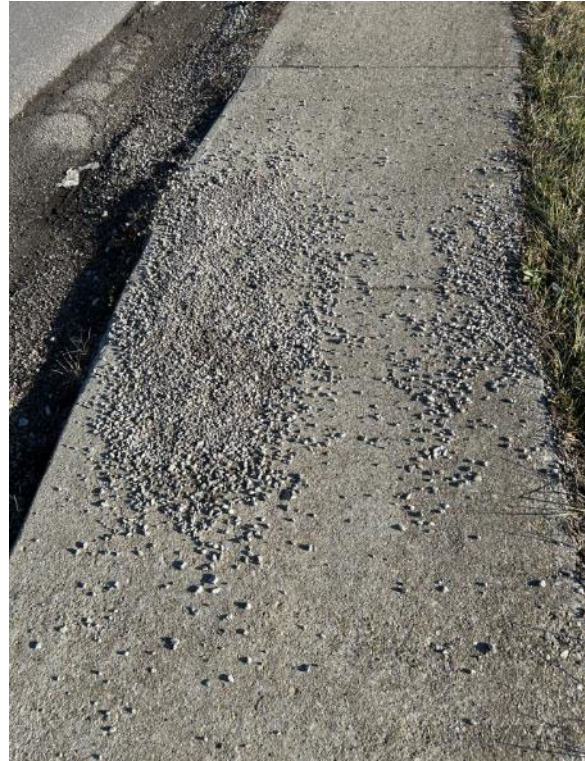
Area with loose gravel on concrete that creates an unstable surface for pedestrians
