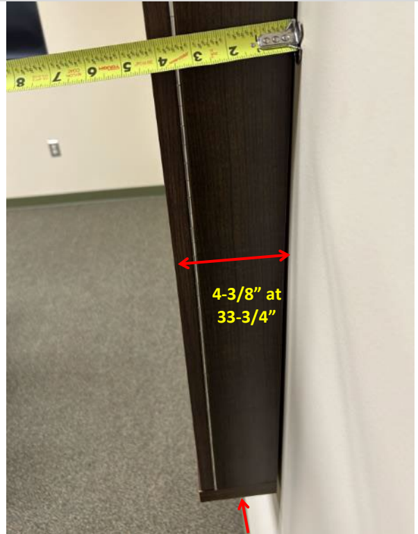
Item #37 White board cabinet protrudes >4"
