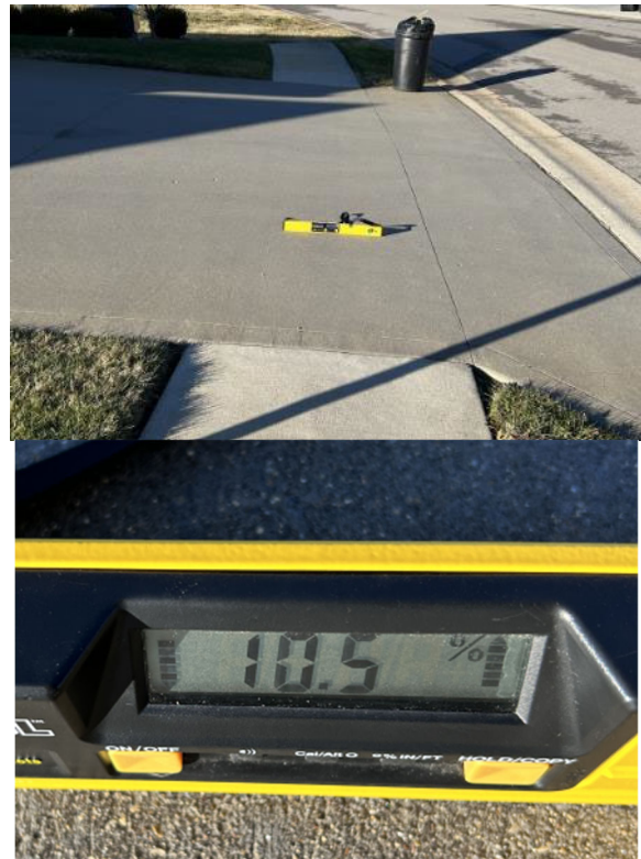
Example driveway with excess PAR cross slope
