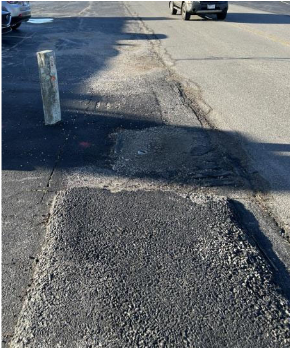
PAR through a driveway that has been patched and presents slope and vertical elevation changes
