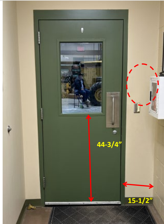
Item #38, 43-44 Entry door in front hallway with no signage, vision light >43" high, latch pull side clear space <18"
