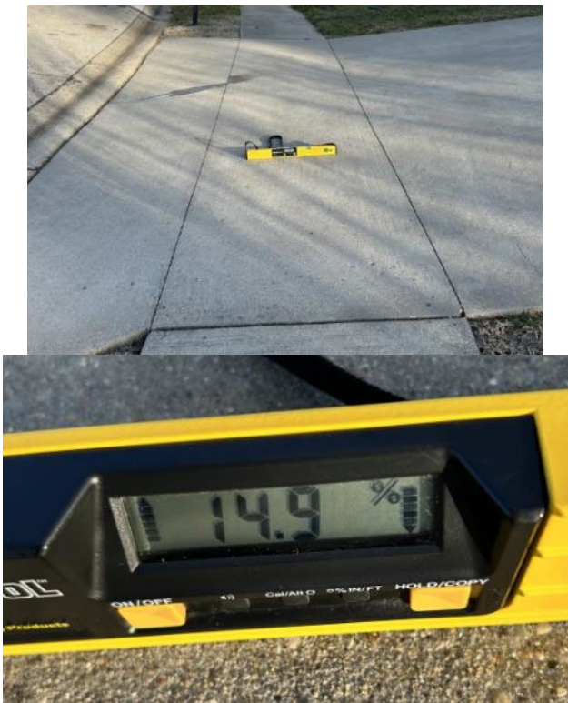
Example driveway with excess PAR cross slope
