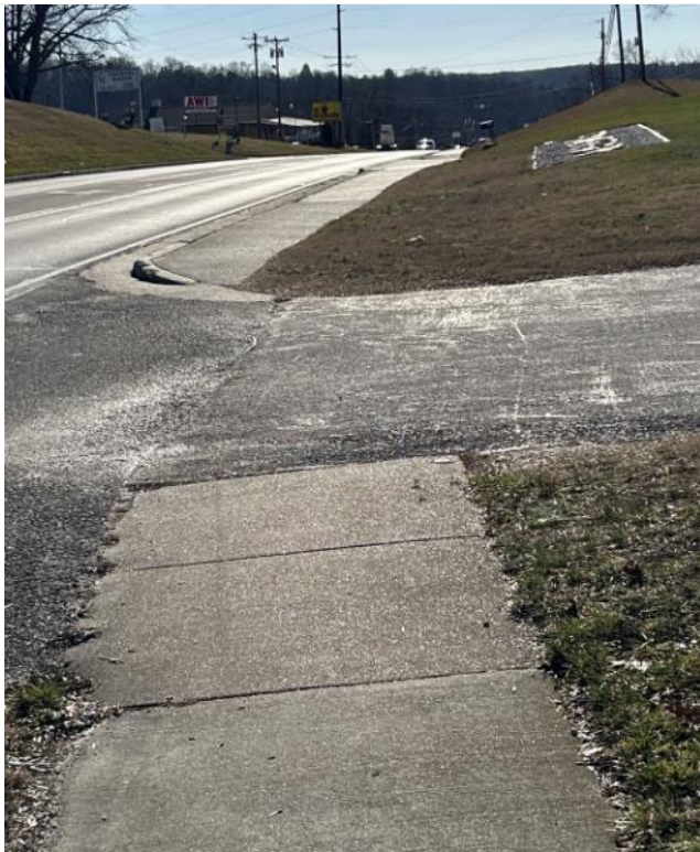
Driveway built through the PAR with severe slope and no compliant receiving ramp at City boundary
