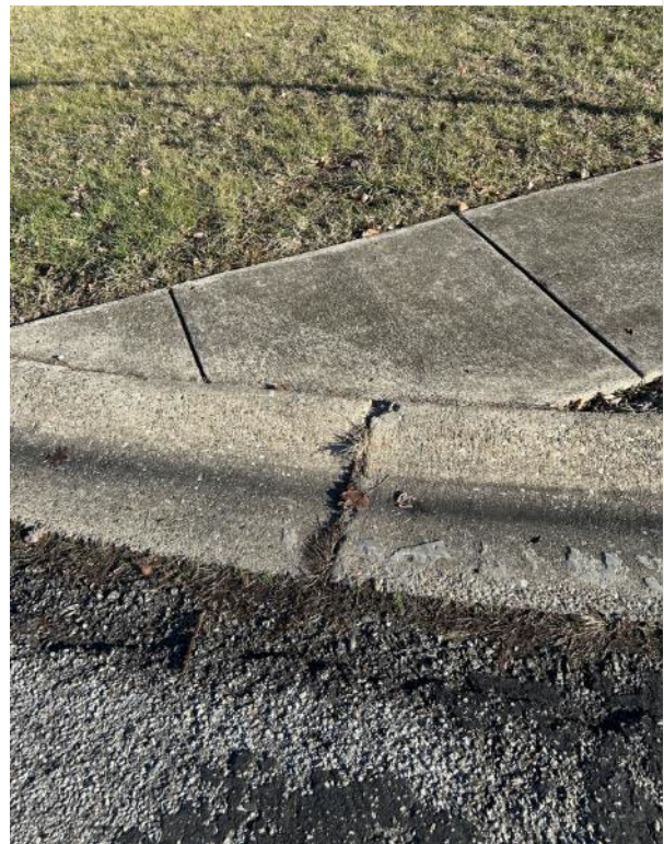
Missing curb ramp at NW end of Settlers Trace
