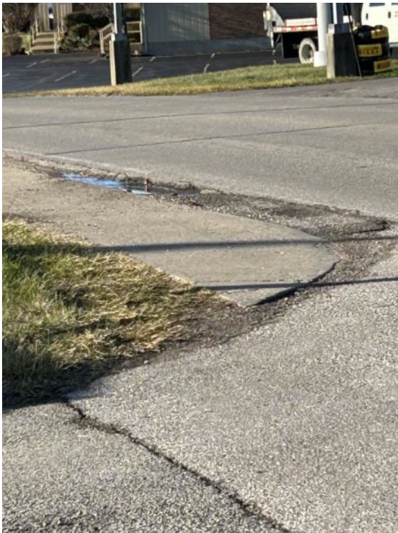
Curb ramp crossing at a driveway with a vertical elevation change
