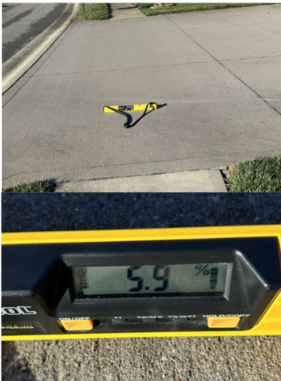
Example driveway with excess PAR cross slope
