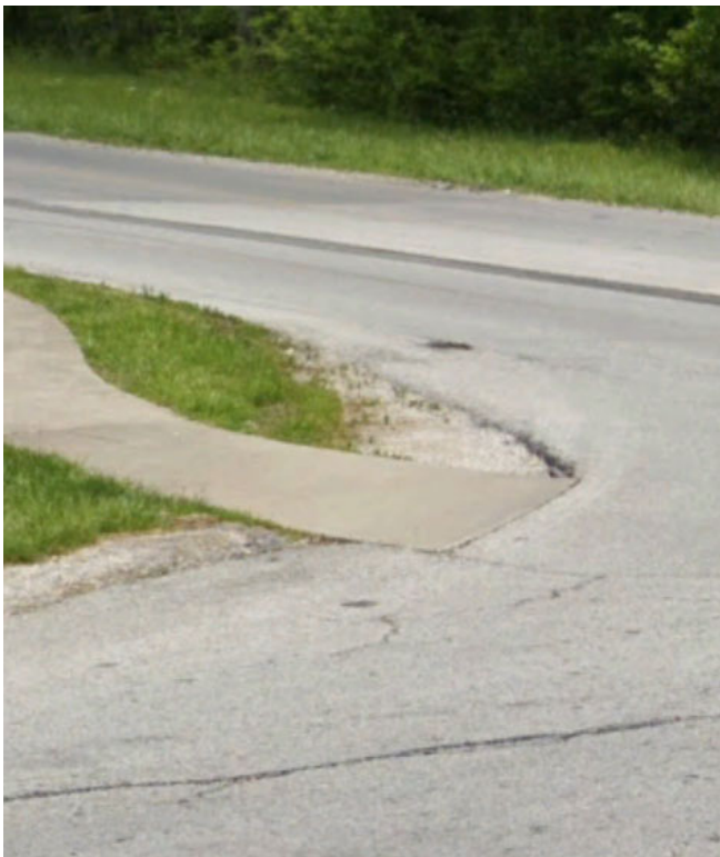
Curb ramp at IN-337 with no DW (Source: Google Earth Streetview)
