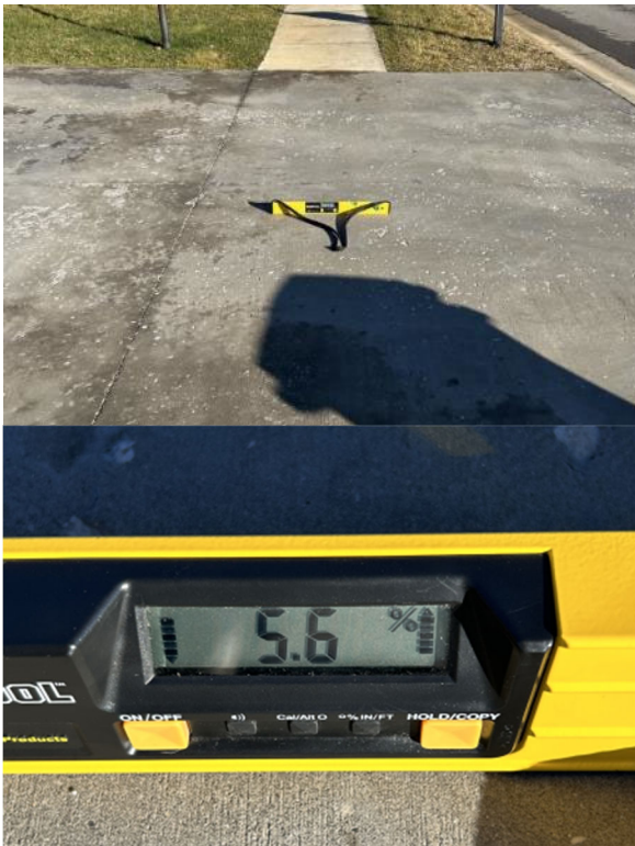
Example driveway with excess PAR cross slope
