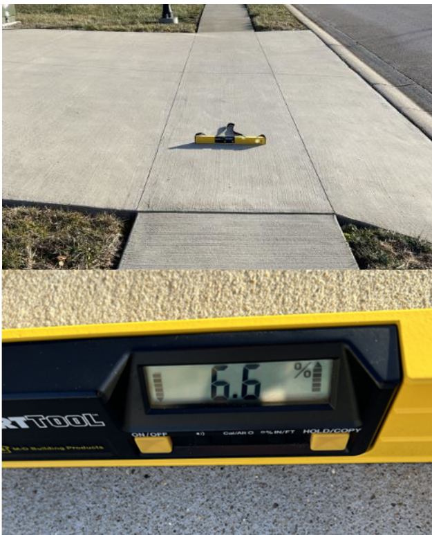
Example driveway with excess PAR cross slope
