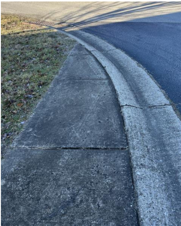
Missing curb ramp at SW end of Settlers Trace
