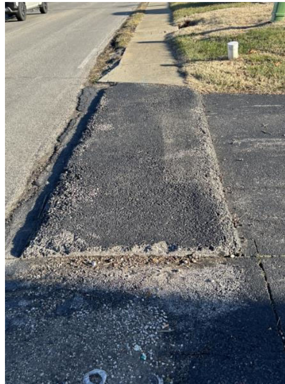
PAR through a driveway that has been patched and presents vertical elevation changes
