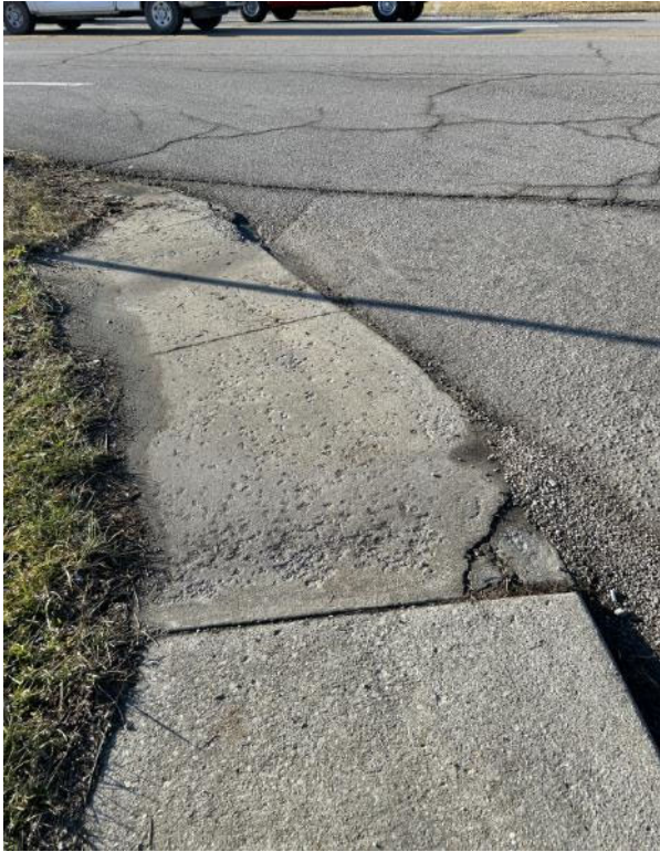
Curb ramp at the southwest end with no DW
