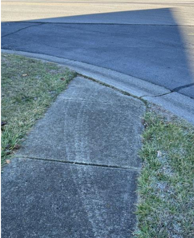
Missing curb ramp at Corydon Ramsey Road NW
