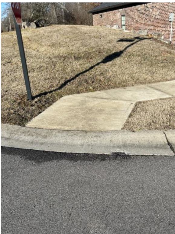
Missing curb ramp at the southwest end intersection of Country Club Road SE
