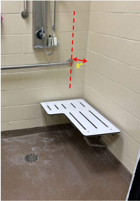
Item #77 Shower grab bar >6" from wall
