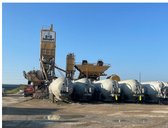
Figure 4-1 Central Mix Plant
