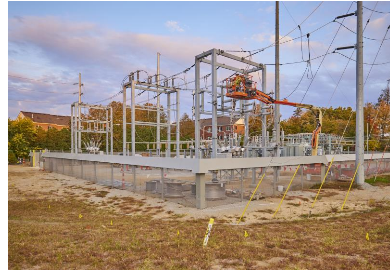
Carmel 69KV Substation
