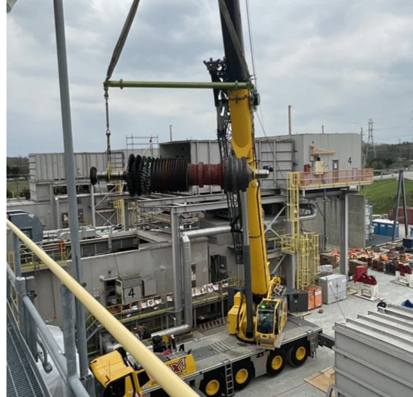
Noblesville Station CT4 – Rotor Lift
