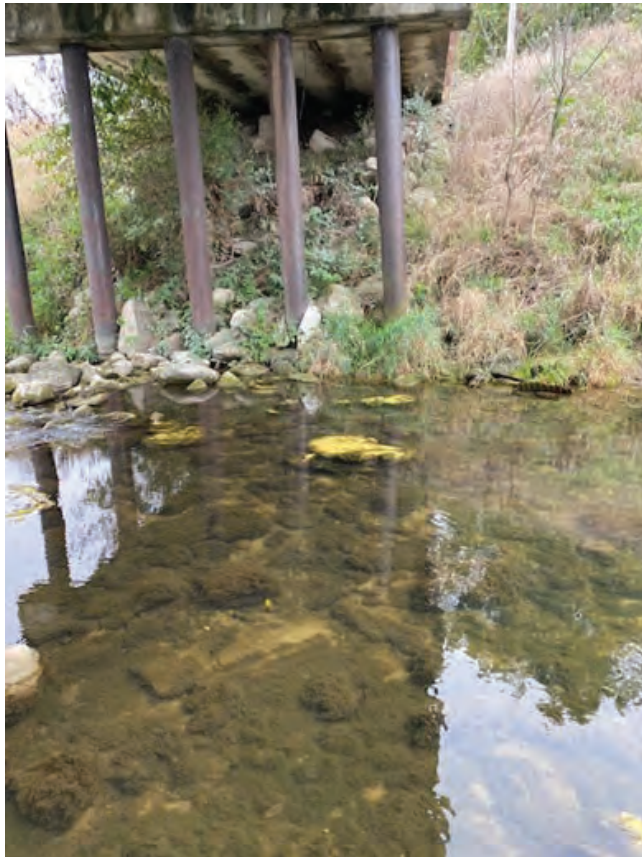
Photograph # 6 under the bridge, looking north across Big Creek Ditch S CR 100 E over Big Creek Ditch, Des. No. 2003033, Bridge Replacement White County, Indiana (Photos taken 10-06-2021)
