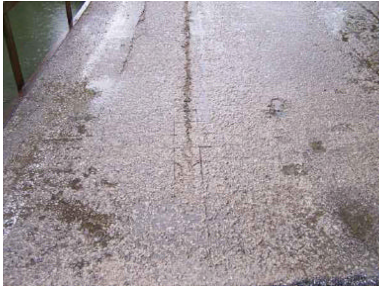
Longitudinal cracks and spalls in deck near southwest corner
