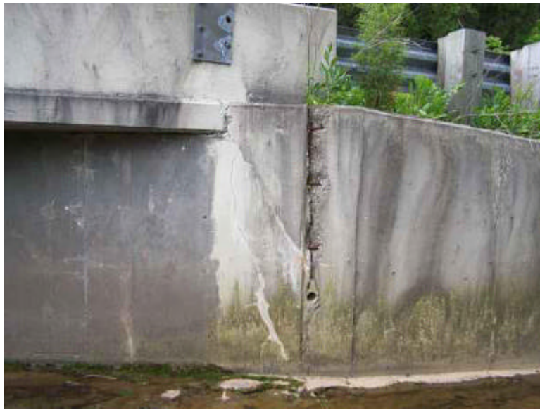
Spalls, cracks & leaching at southwest corner
