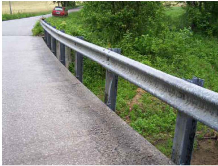
Deck spalls and bent east side bridge railing
