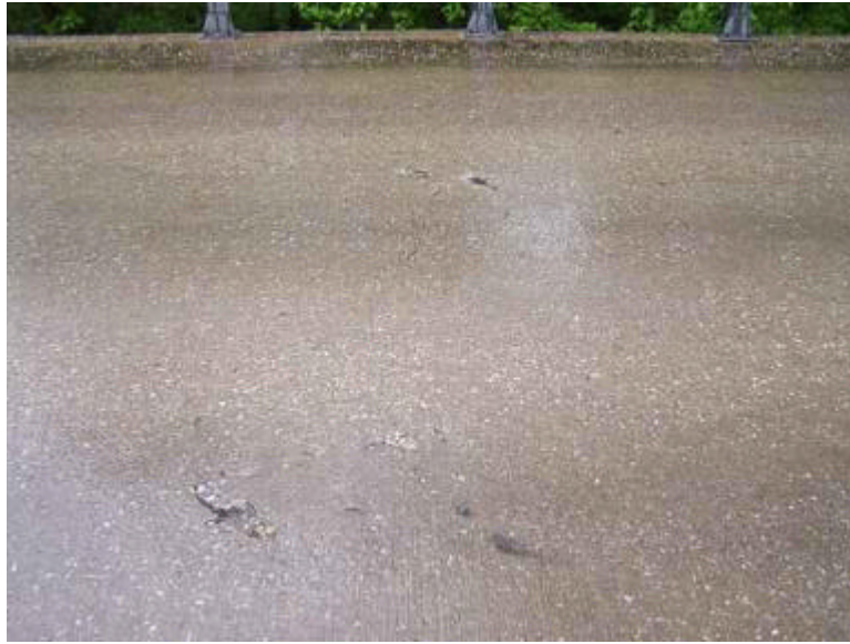
Deck spalls over north pier
