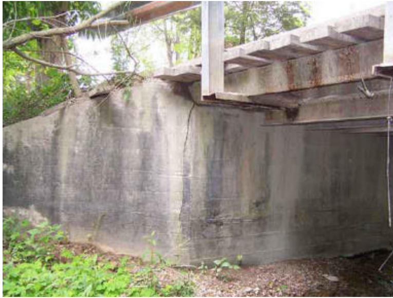
Vertical crack between abutment and northeast wingwall
