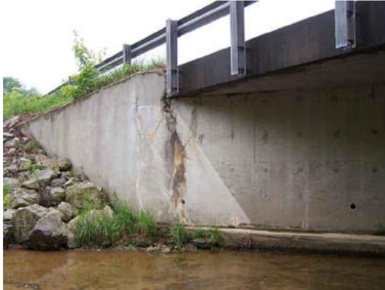
Cracks, spalls & leaching at northeast corner
