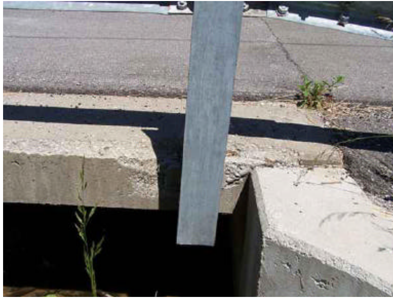
Spall at railing post connection
