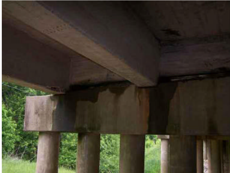
Deck drainage onto pier Spall on bottom of outside tee beam
