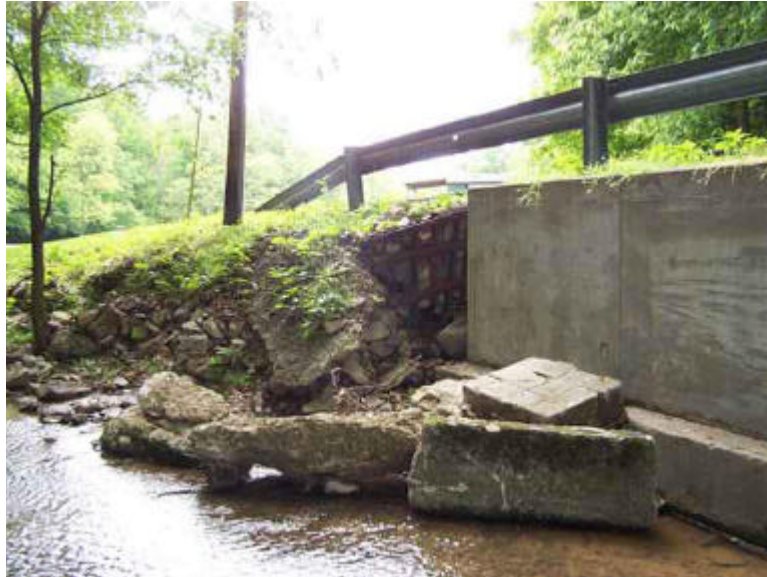
Large concrete chunks in channel beside southeast wing
