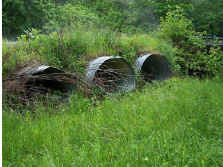
Corrugated metal pipes placed under approach roadway starting approximatel 19 feet from east end of bridge
