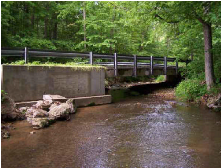
Poor stream alignment and debris in channel
