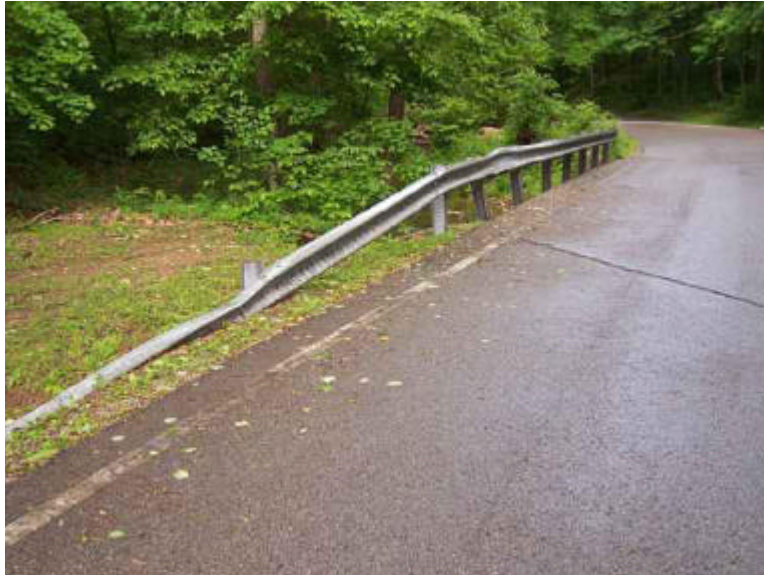
Guardrail damage in southwest quadrant
