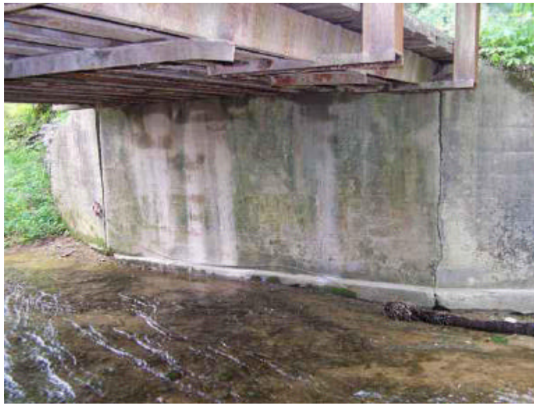
Vertical cracks between abutment and wingwalls
