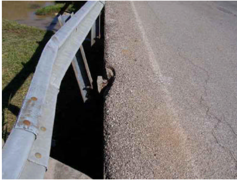
Damaged bridge railing at southwest corner
