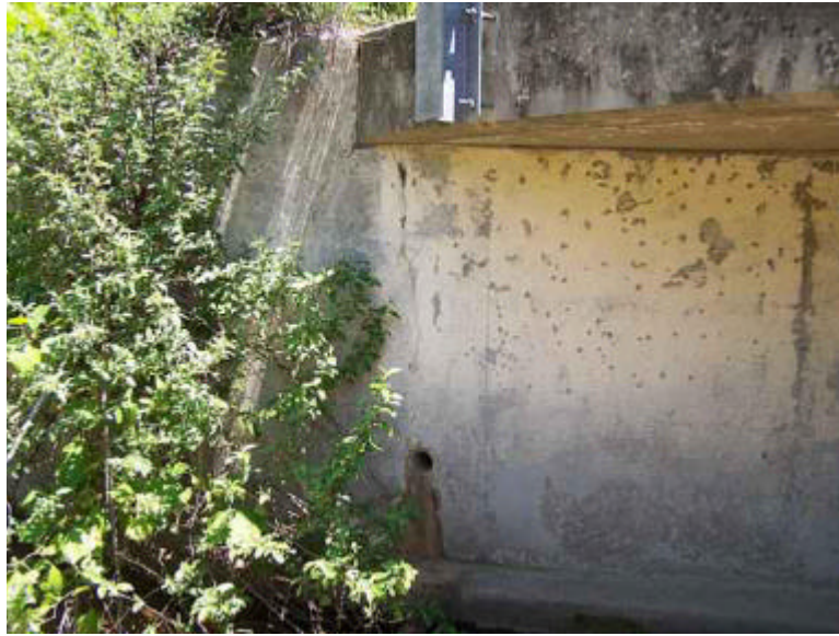
Vertical hairline cracks near north end of east abutment
