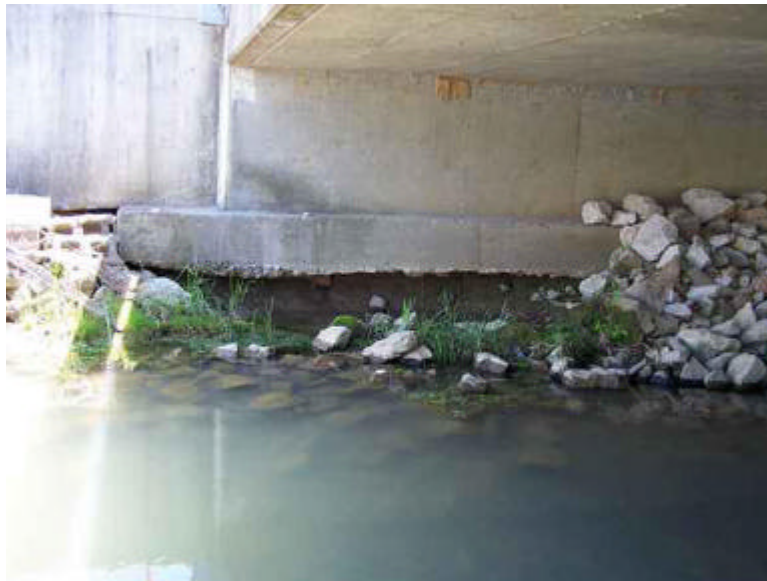
Undermined north end of east abutment
