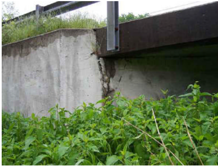
Abutment cracked and spalled at southwest corner
