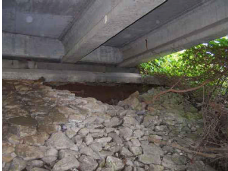
erosion under northeast corner
