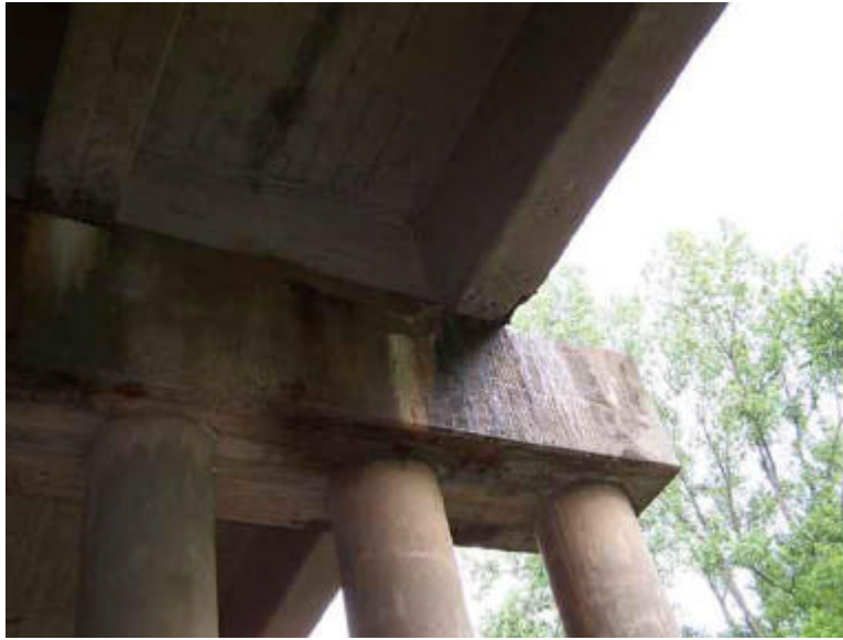
Spalled pier cap with exposed rebar
