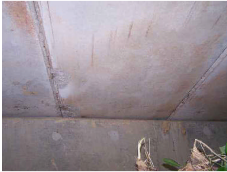
Spalls on bottom of fourth beam from west at north end
