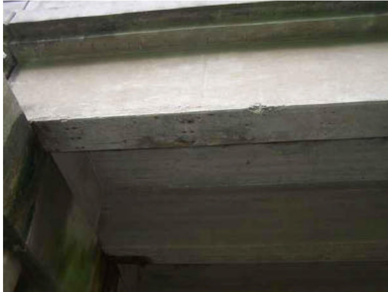
Spalls on bottom of concrete tee beam
