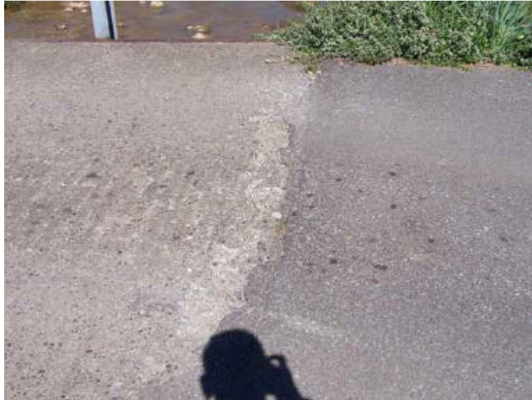
Deck spalls on east end of bridge
