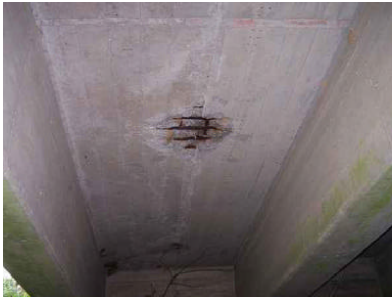
Large spall in bottom of concrete tee beam
