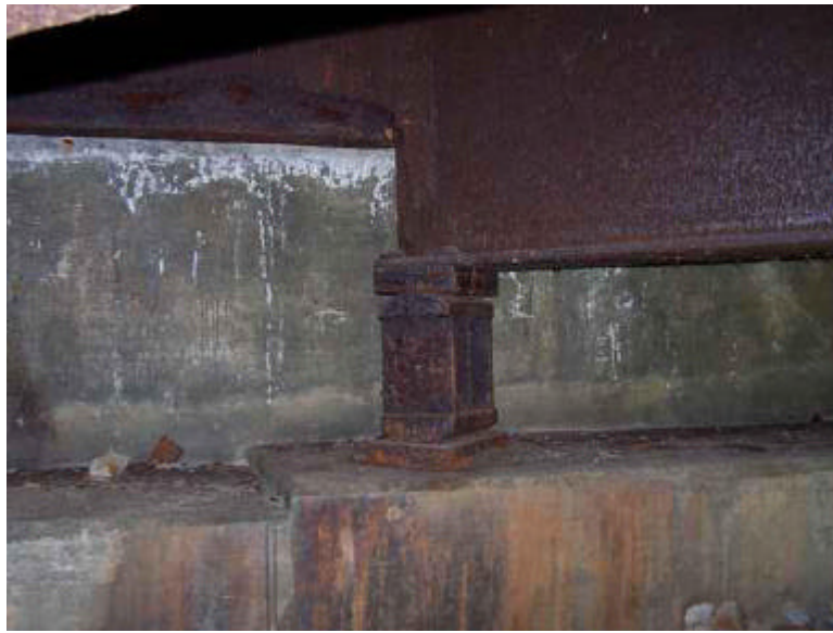
Heavy rust on north bearings
