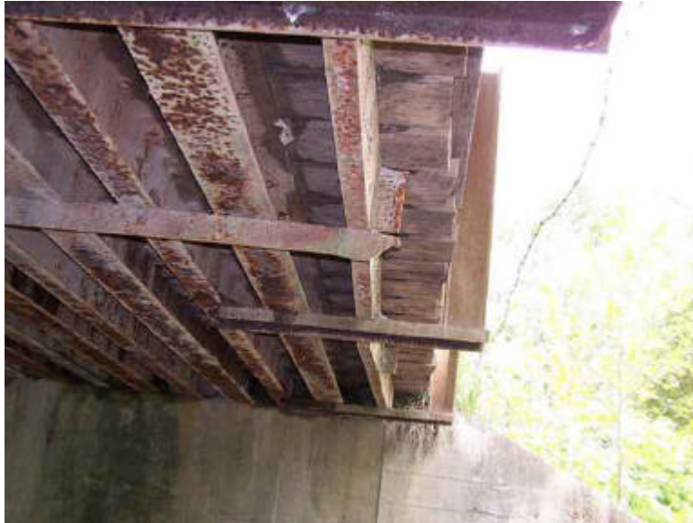
Channel beam under east coping is bent and twisted
