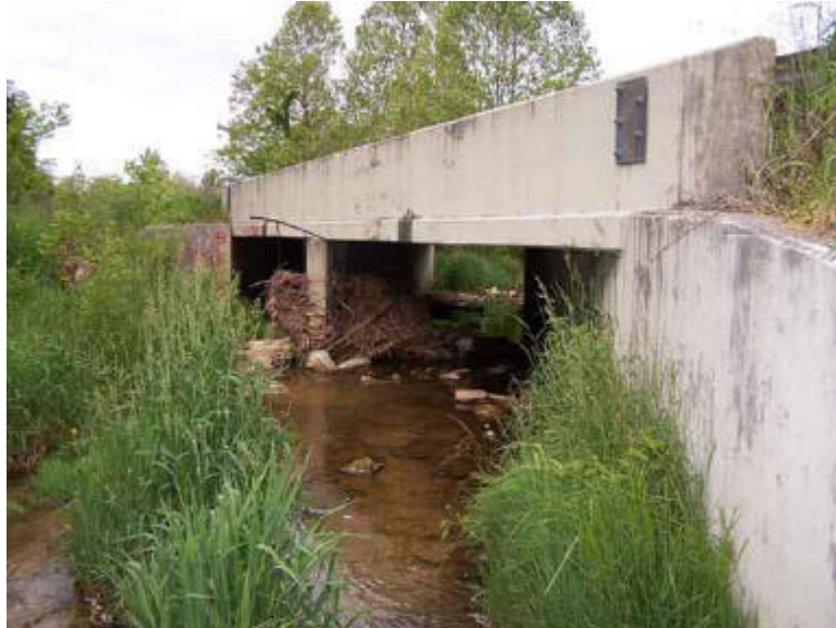
Drift jam lodged on pier
