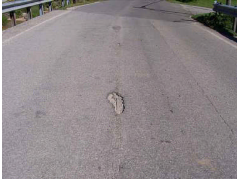
Spalled wearing surface
