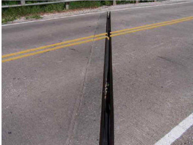
Damaged expansion joint at south end bent
