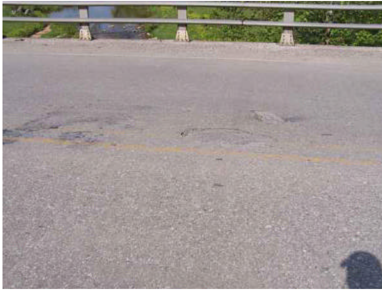
Deck spalls near middle of center span
