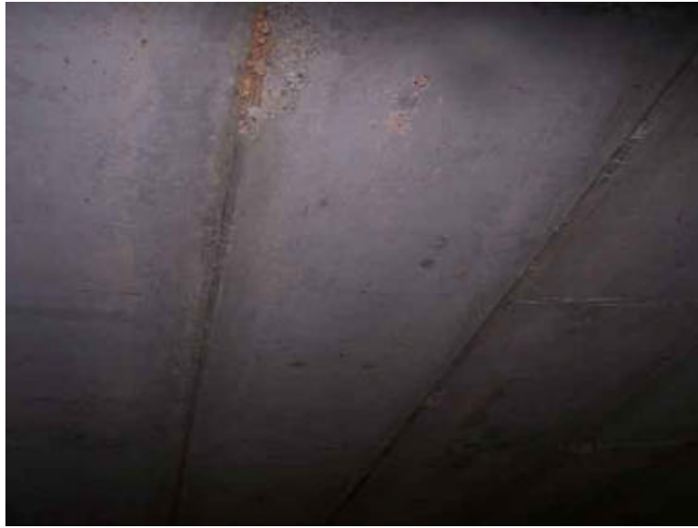
Small spalls on bottom of beams
