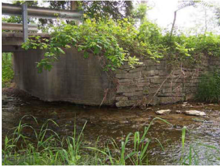
Undermined southeast wingwall
