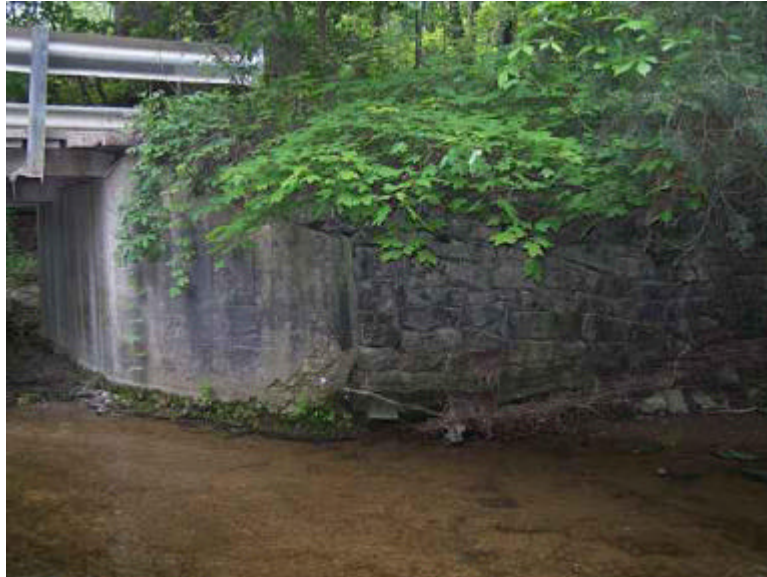
Stone wall extending northwest wing partly undermined
