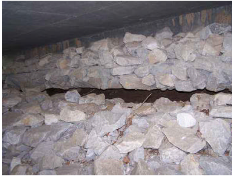
Riprap sliding down north spill slope
