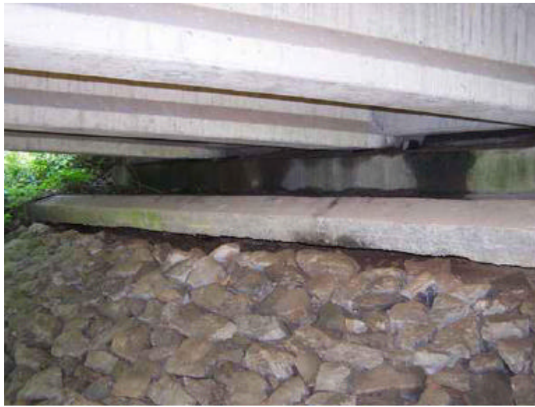
Undermined curb along south end bent
