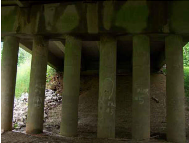
Spalls on cap and pile encasements of east pier Riprap in eroded ditch under east span
