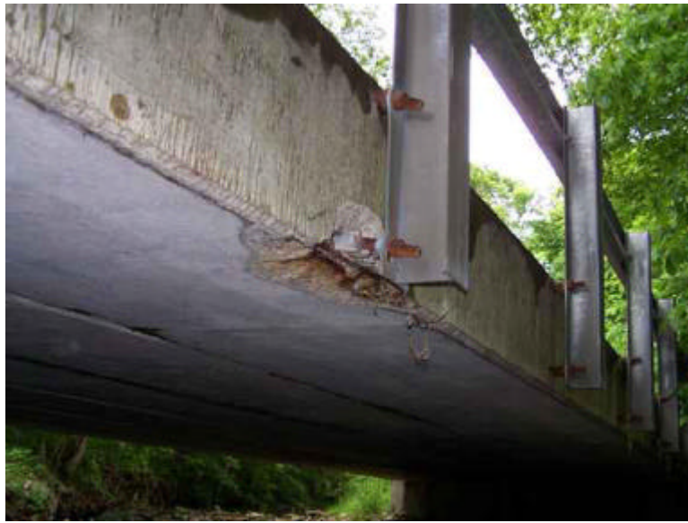
Beam spalled at railing post connection
