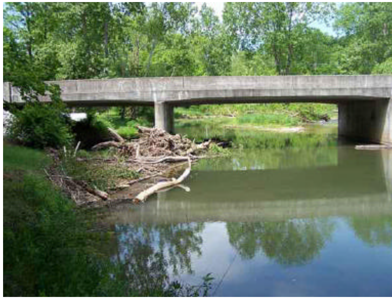
Drift jam lodged on south pier
