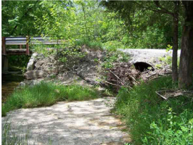
Drift lodged at inlet end of corrugated metal pipe placed under north approach roadway
