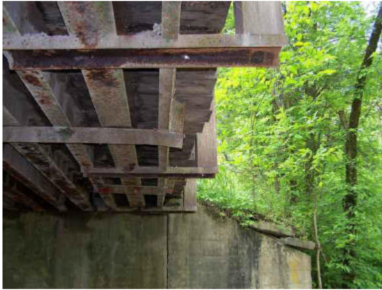
Twisted channel beam under west coping
