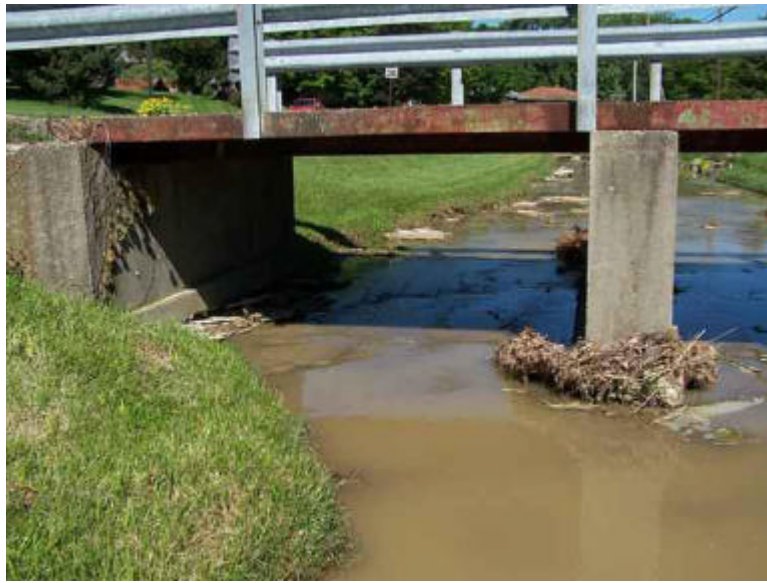
Small drift jam on east end of pier
