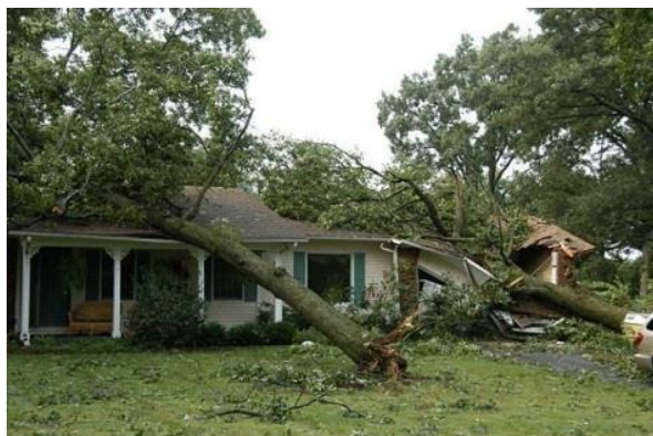
Figure 3-15 Home Damaged During Windstorm
