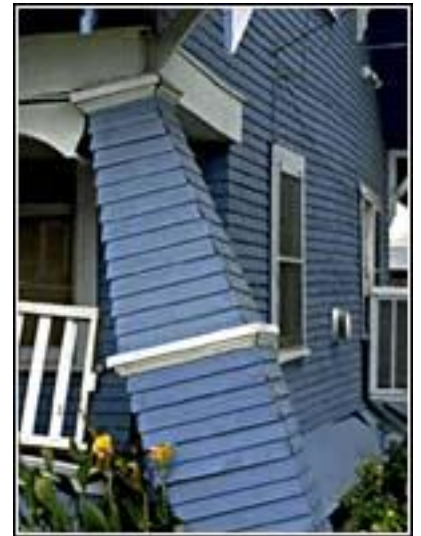
Figure 3-6 Earthquake Damaged Porch
