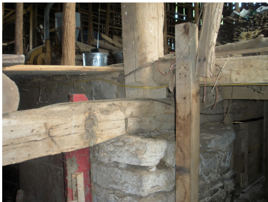
Figure 11. Anderson barn interior showing timber construction typical to hay press barns: stone foundation, horizontal sill with a shiplap connection, and a vertical post. Photo courtesy of Christopher Baas.
