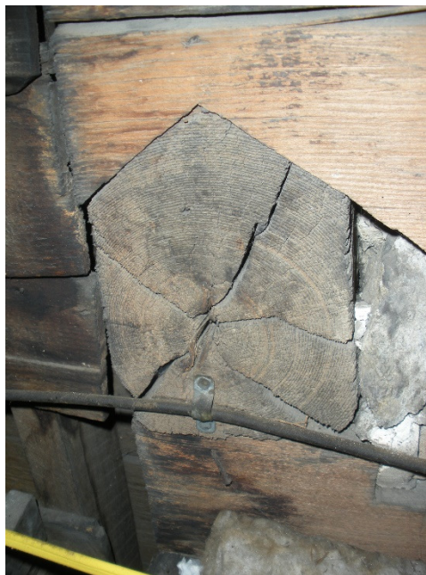
Figure 15. Anderson house corner V-notch located in the roof space over the porch of the original log structure. Photo courtesy of Christopher Baas.
