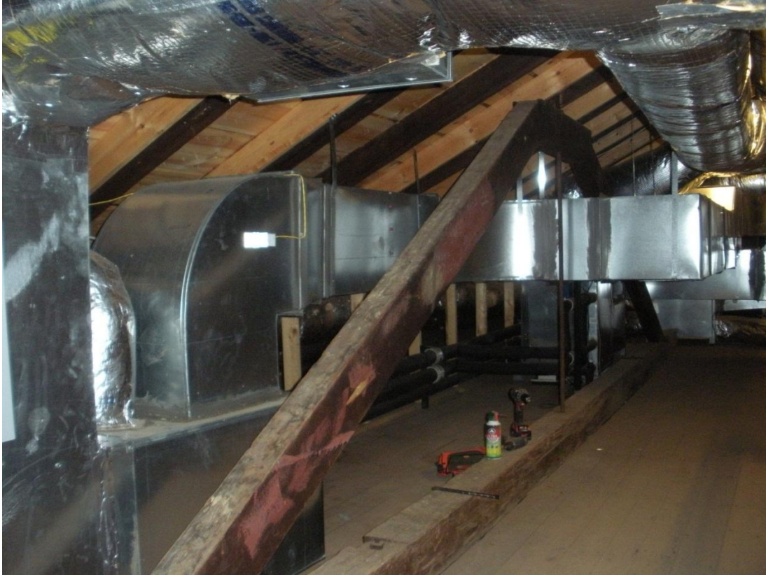
Figure 9. West attic truss looking north. Roof rafters are visible behind the truss and HVAC equipment (photo courtesy of Christopher Baas).
