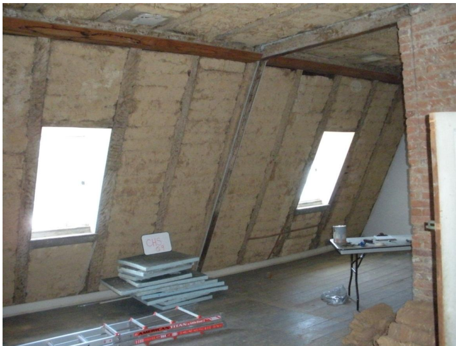
Figure 6. Third floor central space looking southeast at east wall. The exposed wall shows the angled framing timbers of the mansard roof, with Dutch biscuits in between (photo courtesy of Christopher Baas).
