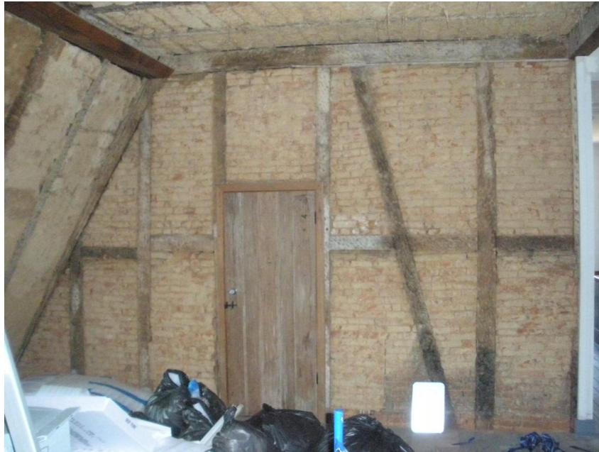
Figure 5. Third floor central space looking north. The exposed wall shows vertical and horizontal timber construction, and angled bracing. The framing is filled with low-fired bricks (photo courtesy of Christopher Baas).
