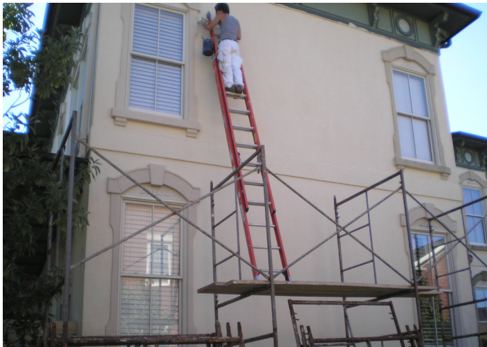
IOSHA Top Ten Most Violated Standards, number 2, Scaffolds. (Submitted Photo)
