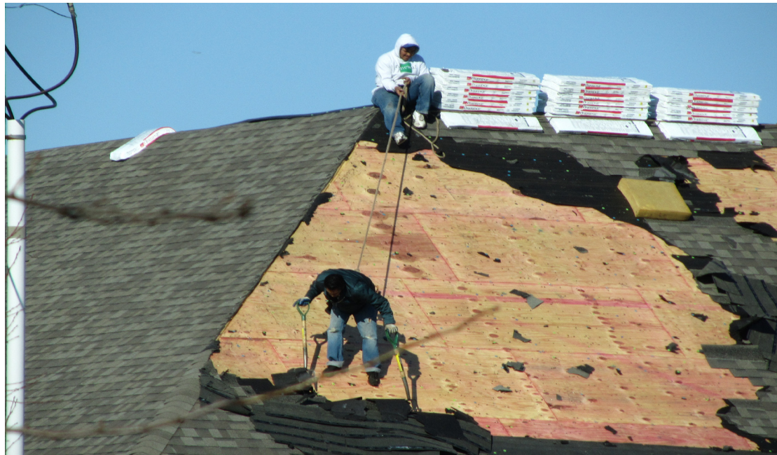
IOSHA Top Ten Most Violated Standards, number 6, Fall Protection: Employee is not properly protected from a potential fall. (Photo submitted to IOSHA)
