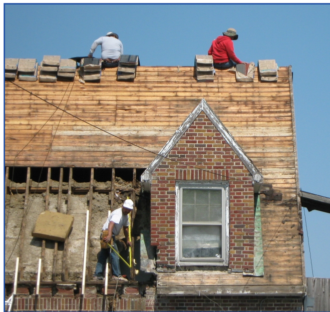
Employees are performing roofing work on a steep pitched roof without fall protection. 29 CFR 1926.501(b)(11). (IOSHA compliance photo)
