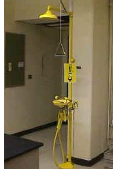
Above: Example of a Safety Shower/Eye Wash Station.
