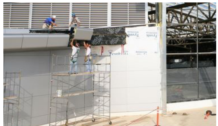
Above: Scaffolding is used in the construction of the new Indianapolis International Airport (Photo Courtesy of Monomedia, Inc.).
