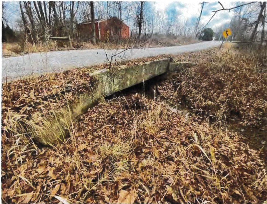
Photo 8. View of the south side of a concrete culvert, construction date unknown, under County Road 700 South facing northeast
