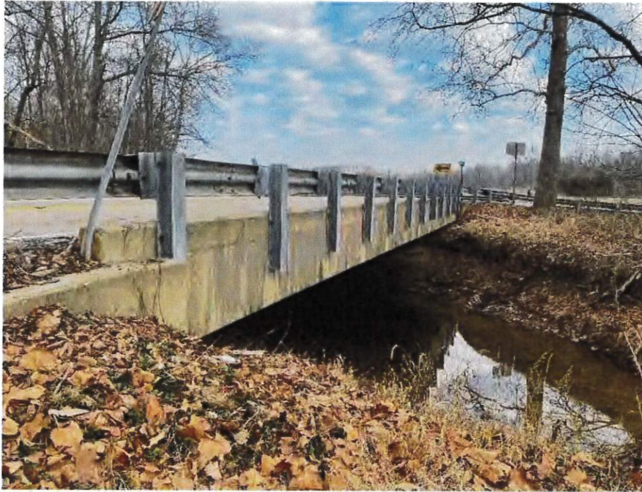
Photo 5. View of south side of Bridge No. 058-03-05882B carrying State Road 58 over White Creek facing northeast
