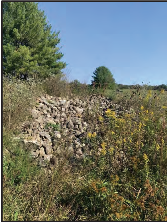
25. View of riprap-lined RSD3 transitioning to vegetated RSD4 located north of SR 258 at the eastern end of the investigated area, looking north. 9/28/2021
