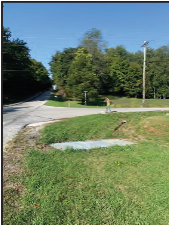
22. View of mowed ROW and drainage inlet on the north side of SR 258, looking west across N CR 100 E. 9/28/2021
