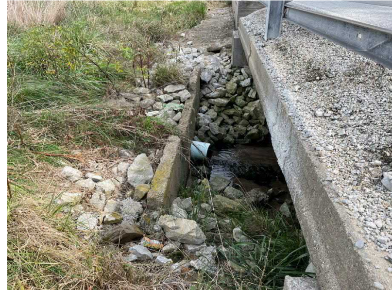
Photo 6. Facing east towards an agricultural field drainage pipe draining into UNT to Koots Fork at the inlet of the project structure.
