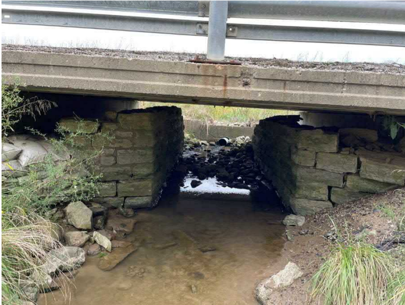
Photo 5. Facing north from within UNT to Koots Fork, looking upstream through the project structure under SR 44.
