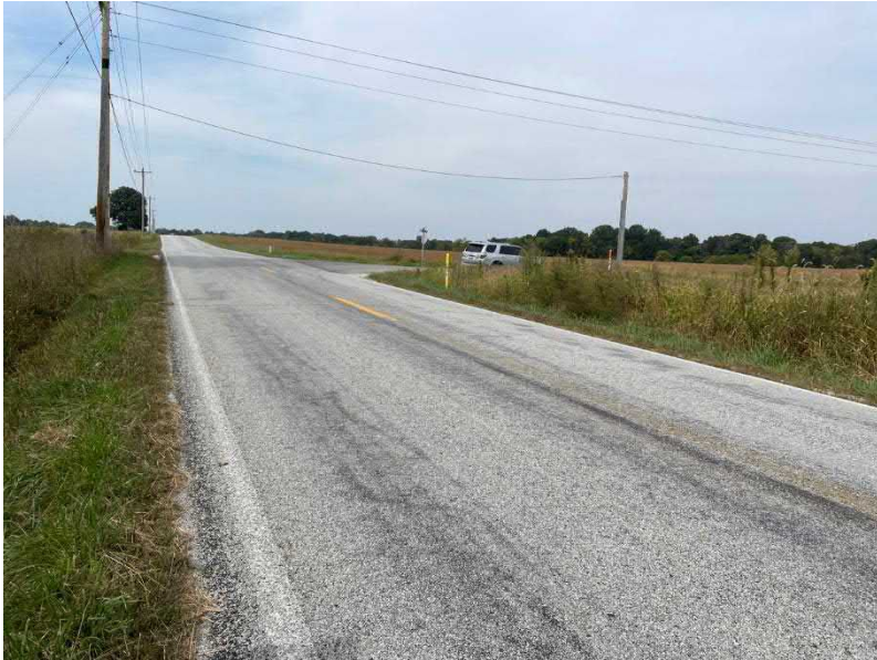
Photo 1. Facing west from the south side of SR 44, looking towards the intersection of SR 44 and CR 575.
