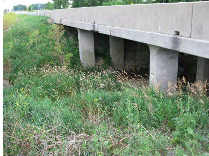
36. Looking northwest at the southern side of the bridge toward Mud Creek.
