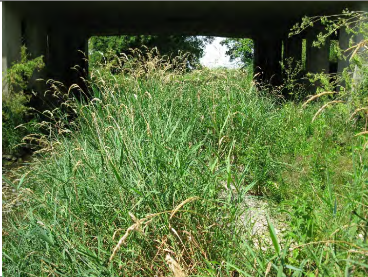
5. Looking north in Mud Creek at an instream wetland feature (reed canary grass) near the south side of the bridge.
