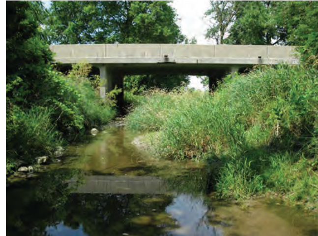
6. Looking north at Mud Creek and US 36 bridge from south side of US 36 bridge.
