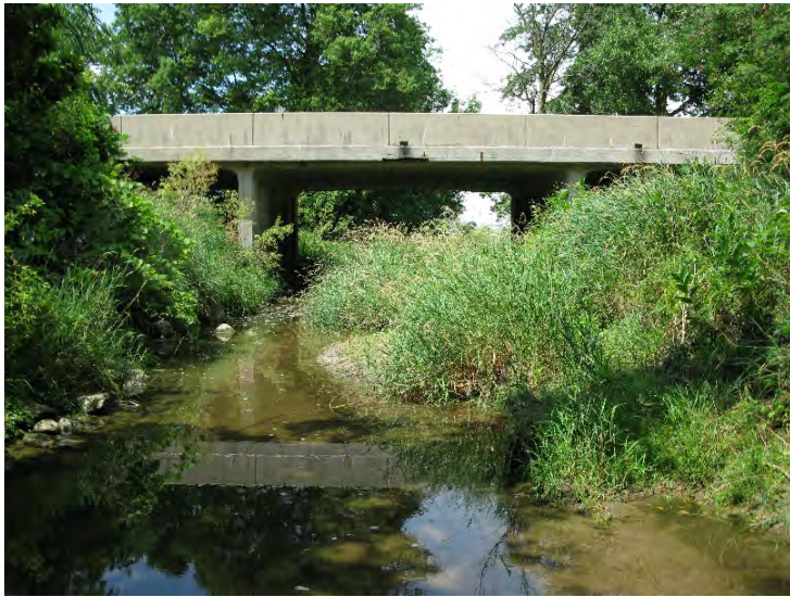
1. Looking north from south side of bridge in Mud Creek. Note instream wetland feature on right.
