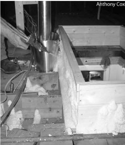
Two-part foam: A contractor air-seals and insulates around an attic hatch dam with two-part spray foam.
