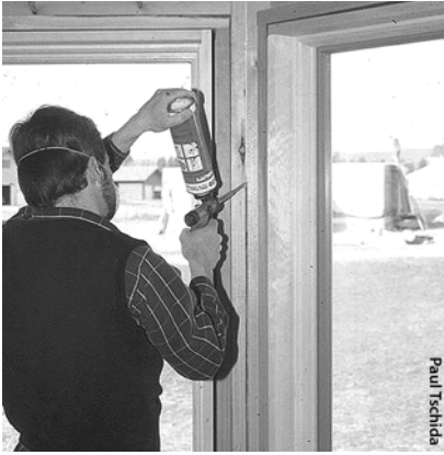
One-part foam: A contractor uses an applicator gun to seal spaces between framing members and around windows.
