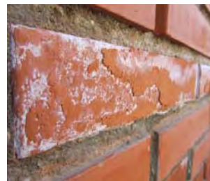
Efflorescence and Spalling
