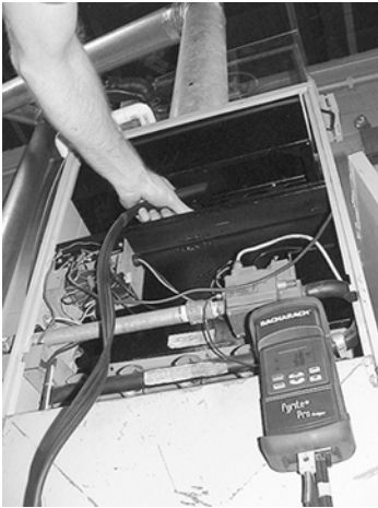
70+ Furnace: Sample flue gases within the draft diverter inside each exhaust port.
