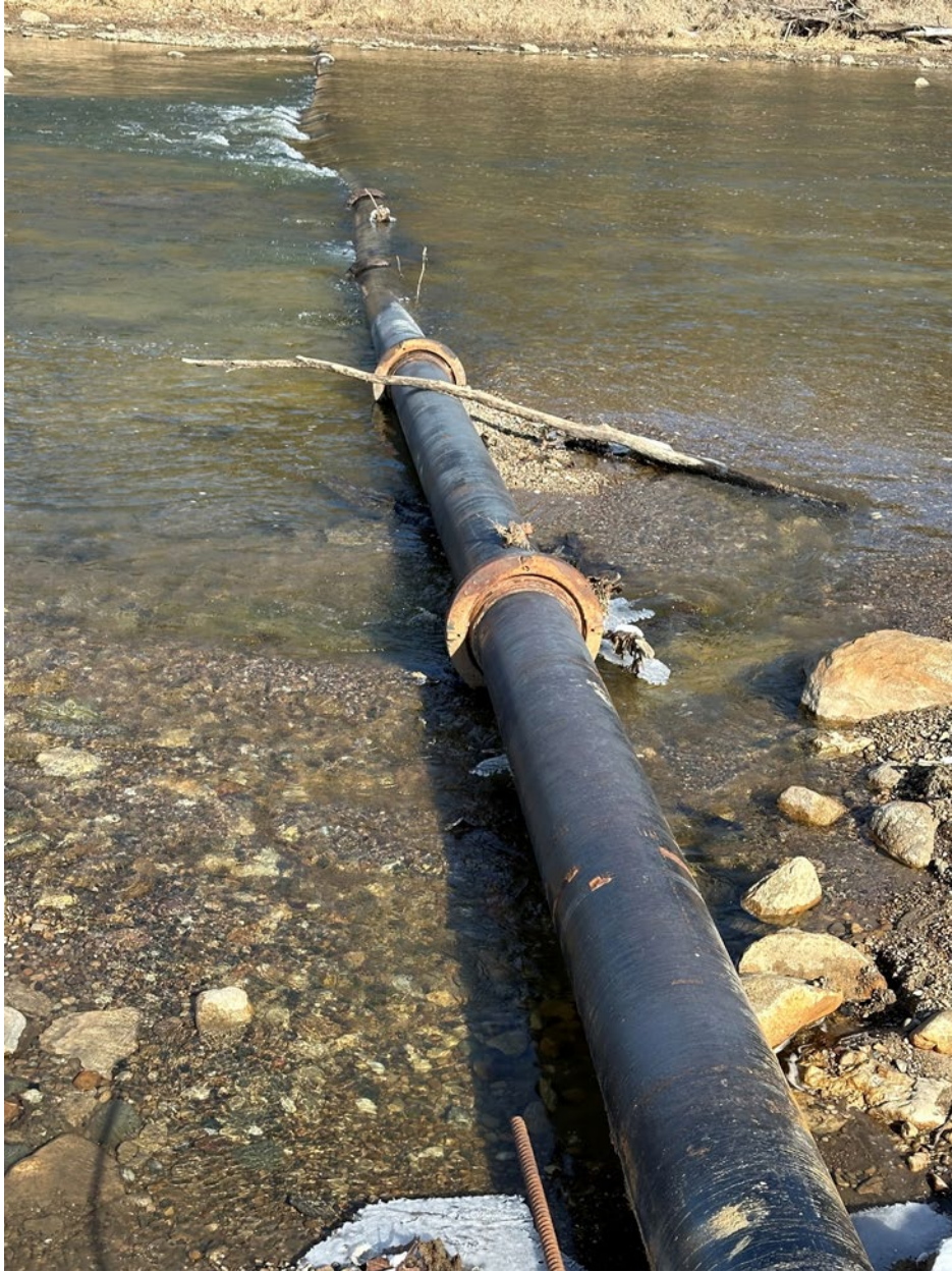
Figure 1. The 16-inch waterline exposed after removal of the low head in November 2021. The dam was 1,280 feet downstream. The waterline is made of castiron and is ½ -inch thick and lined with cement. The pipe joints are made to articulate using a “ball and socket” connecting joint.
