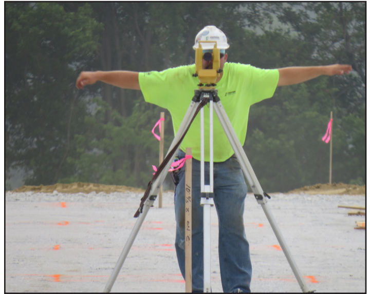
A Pepper tradesman performs layout for the new Gordmans Distribution Center. The 530,000-square-foot warehouse, which is being developed by Ambrose Property Group, was substantially completed in November 2013. (Photo provided by Dave Murphy, Safety Director for Pepper Construction.)
