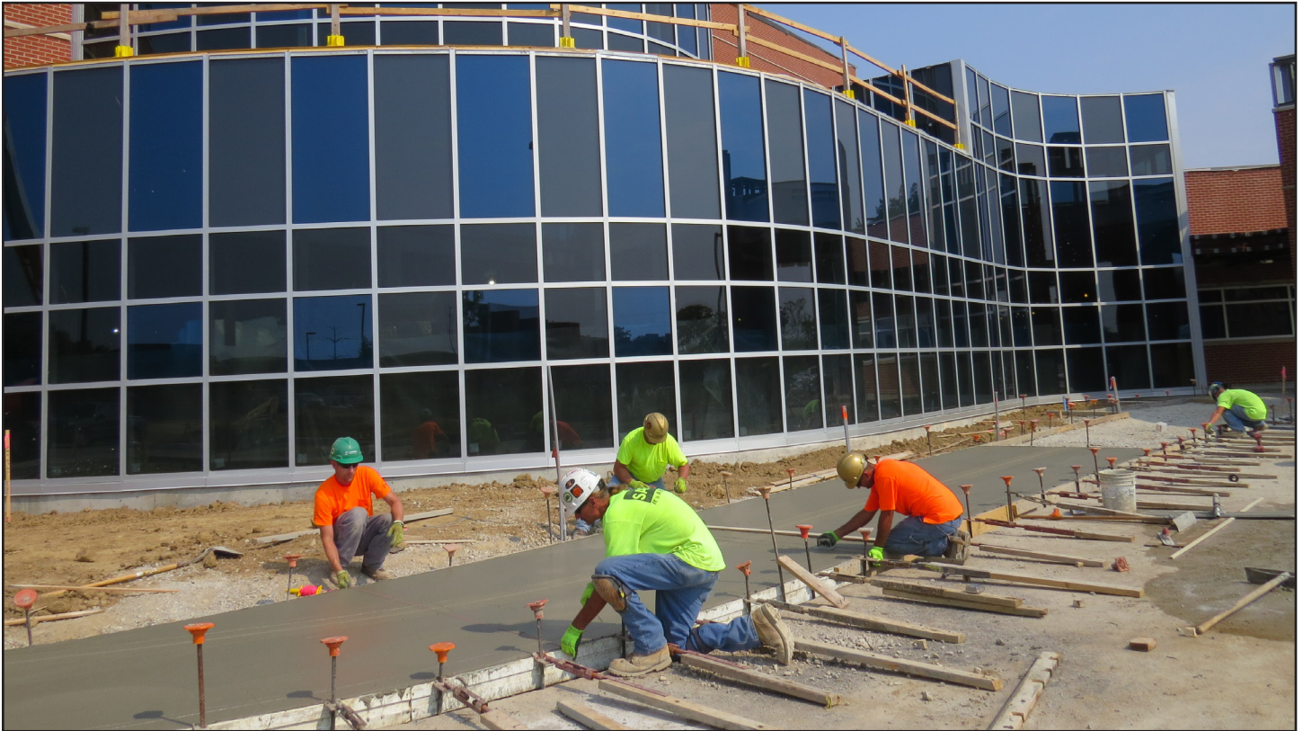
Tradespeople work on hardscapes for new Community Health Network South Regional Cancer Center. The new three-story Cancer Center will open in spring 2014. (Photo provided by Dave Murphy, Safety Director for Pepper Construction.)
