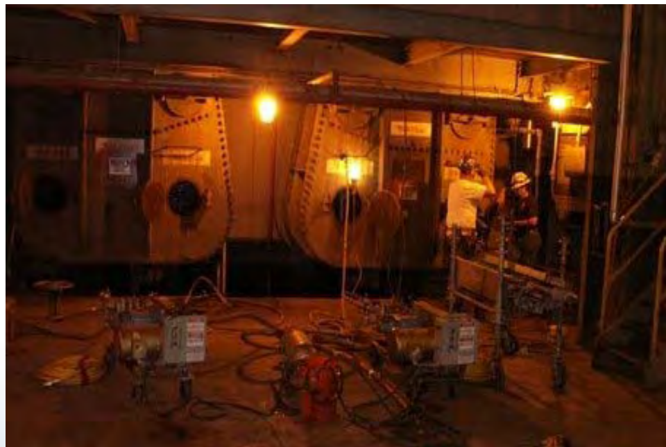
Summer 2010 Preparation: HSS Unit 5 Condensor Cleaning
