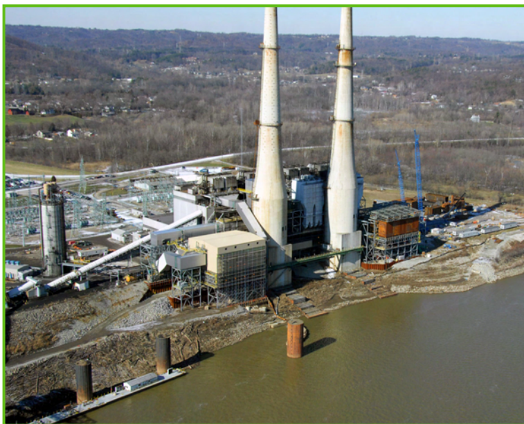
Gallagher Station – January 2008
