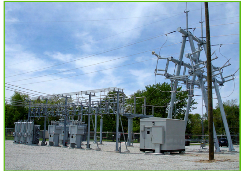
Lafayette Shadeland Substation – May 2008
