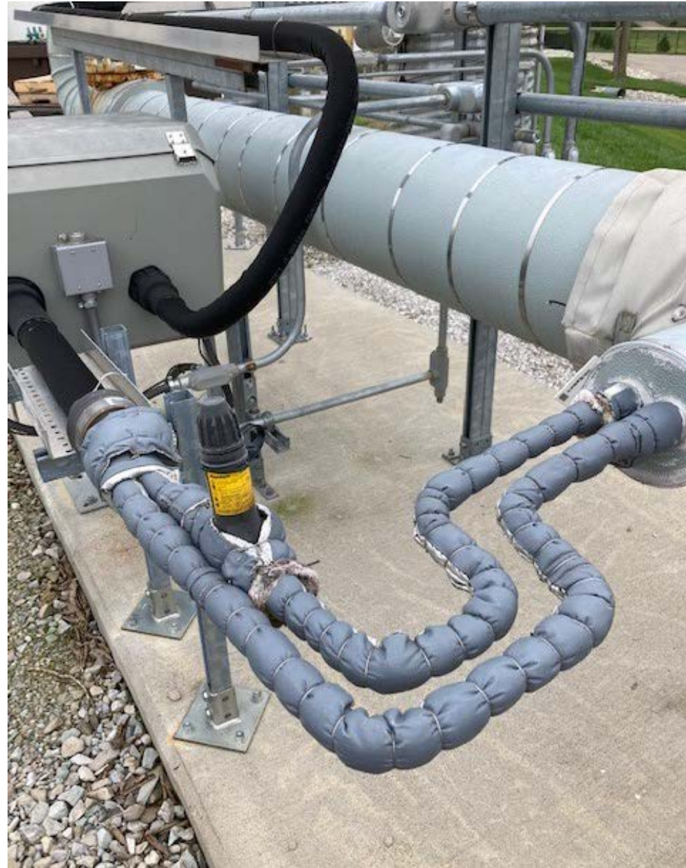
Well Pump Heat Trace
