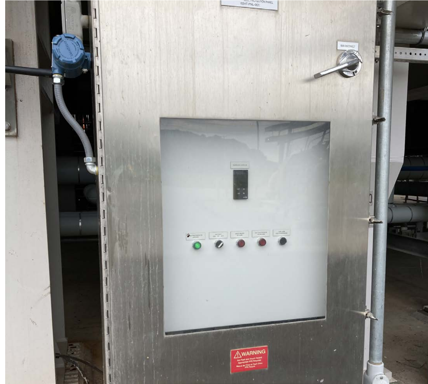
Heat Trace Control Panel
