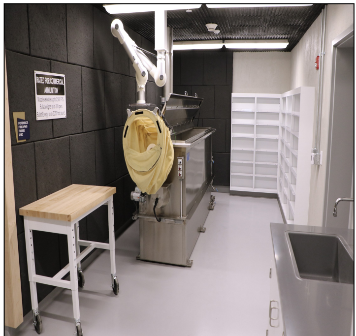
Firearms Unit Laboratory including a water recovery tank
