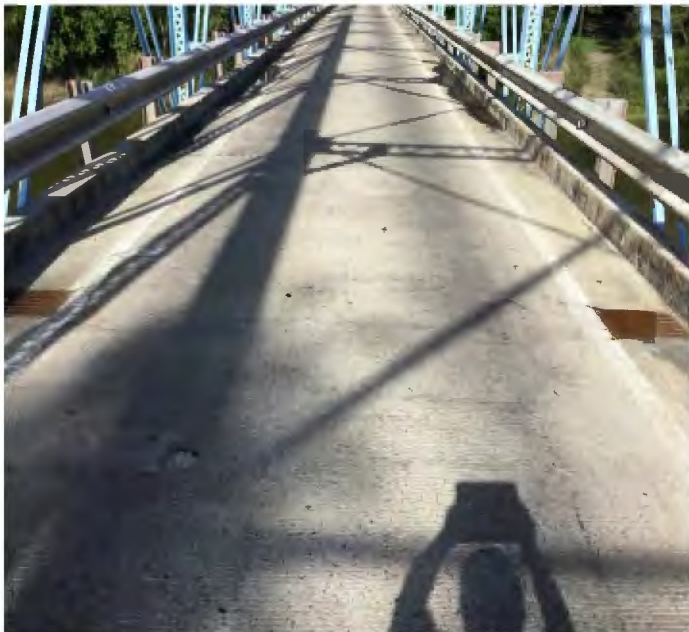
PHOTO 4 Description Span C with many spallings
