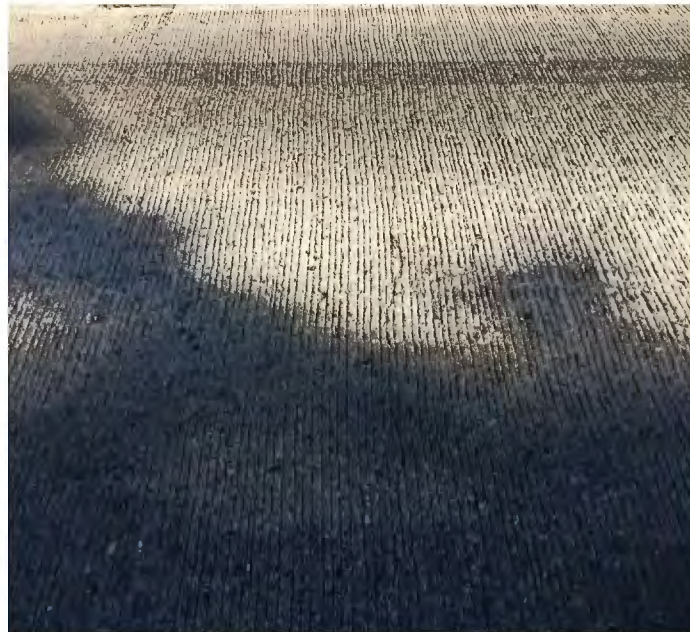
PHOTO 6 Description Span D wide width transverse cracks at 5 feet apart
