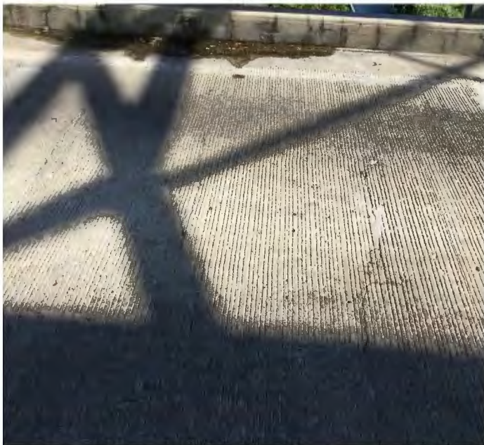
PHOTO 3 Description West end of Span B with more patching and cracks
