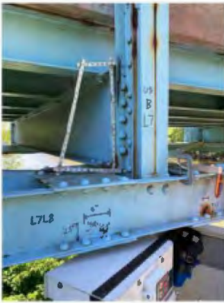
File Description US Span B, U7L7, 0.25" crack in interior angle flange, 20" from the bottom of the vertical pic 1
