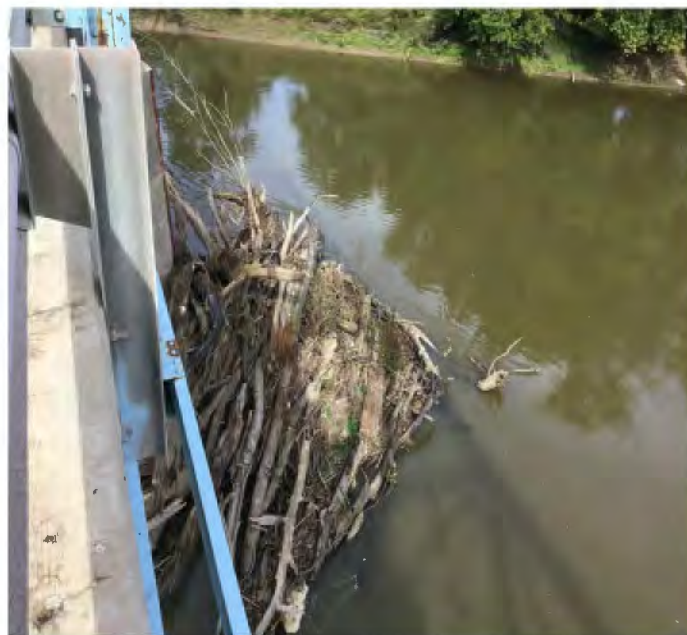
PHOTO 2 Description Look north at east side of Pier 2 log jam
