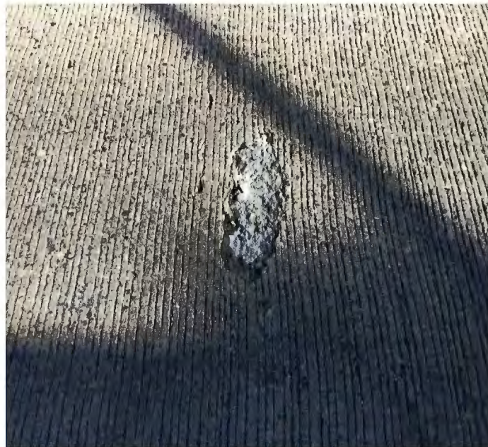
PHOTO 5 Description Spalling at mid span D
