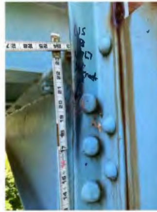
File Description US Span B, U7L7, 0.25" crack in interior angle flange, 20" from the bottom of the vertical pic 2
