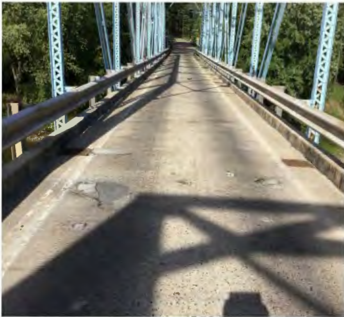
PHOTO 1 Description Span A with patching and spalling
