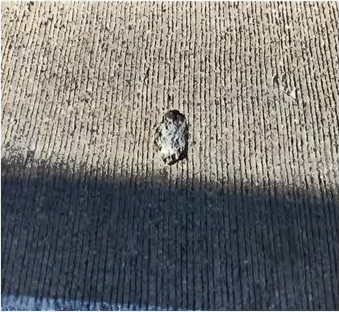
PHOTO 7 Description Spalling at north end of span D
