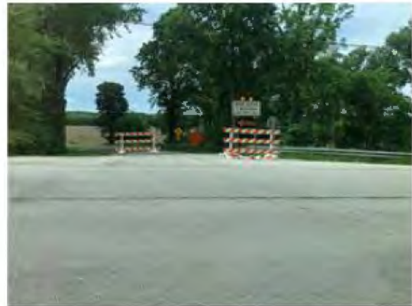
File Description Road Closure Signage at Old SR 25 and SR 225 File Type Category CF Closeout
