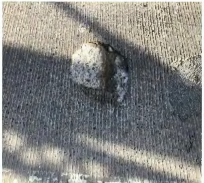
PHOTO 2 Description Span A with delamination and exposed rebar
