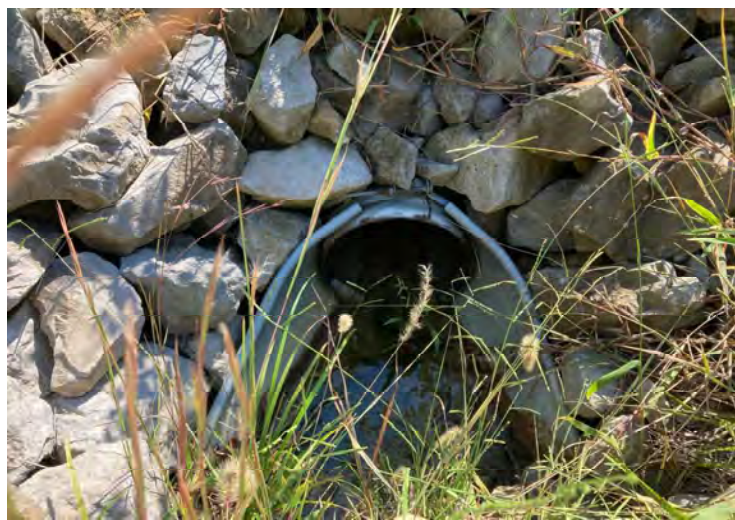
12 – View of corrugated metal pipe inlet facing southeast - Pipe connected to RSD2 - No work being done on pipe
