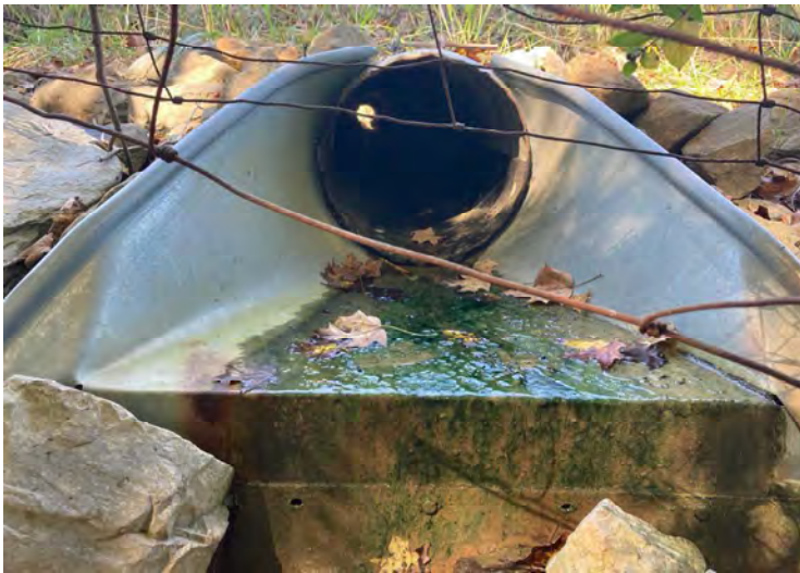
14 – View of corrugated metal pipe outlet facing northwest - Pipe connected to RSD2 - No work being done on pipe
